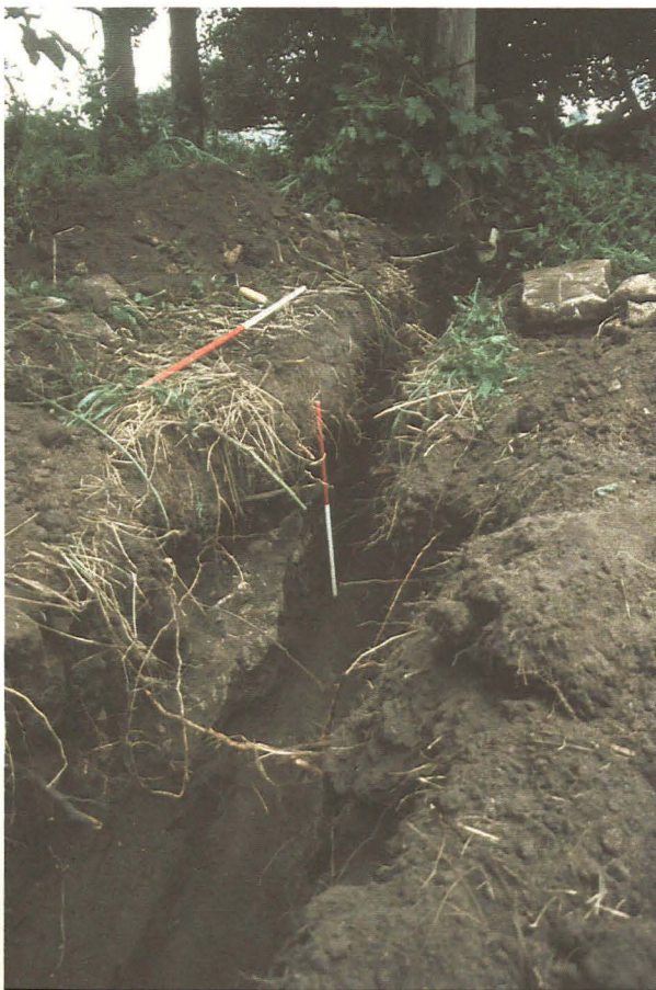
▲ Plate 1 General view of Dutch Cottage yard prior to excavation of the cable trench.
