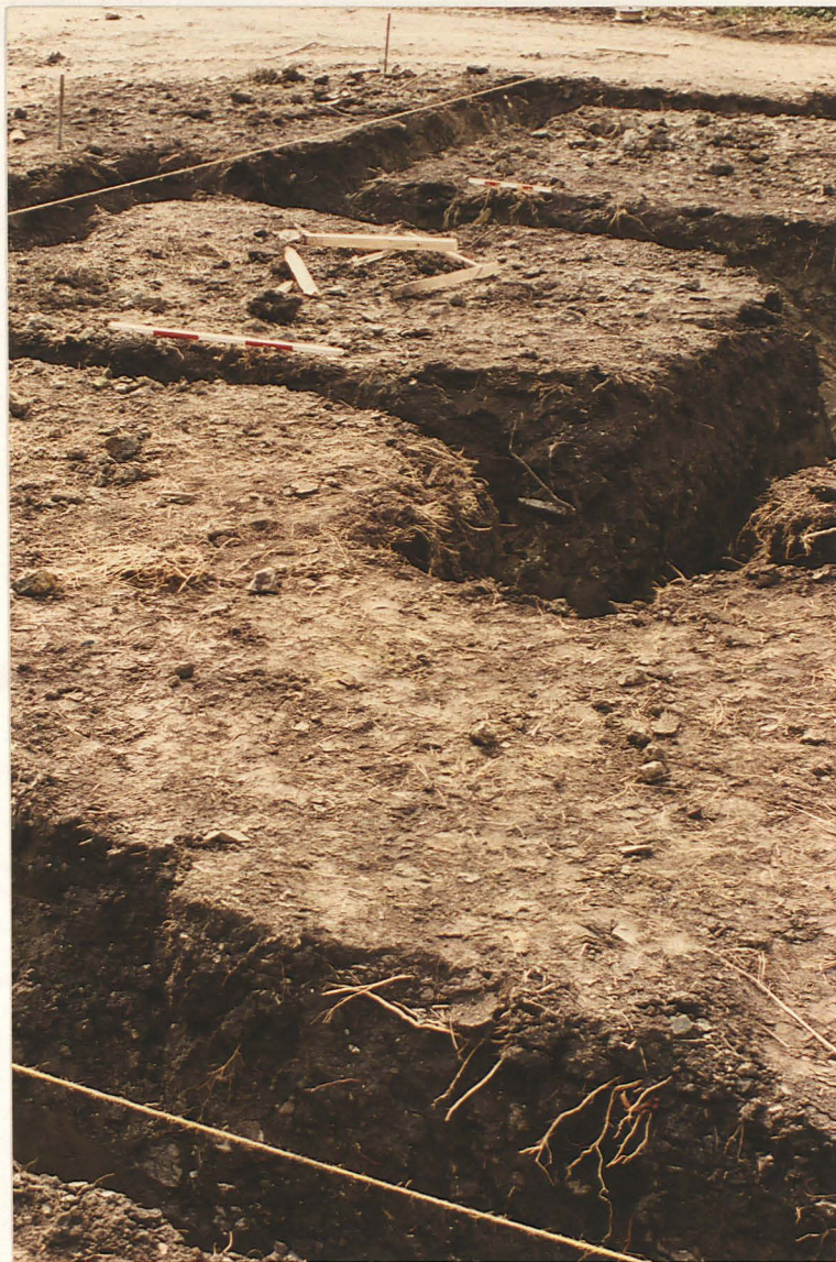
Pl. 13 Position of gully marked by scales cut by the house foundations (observation 9 centre, observation 8 rear, looking west).
