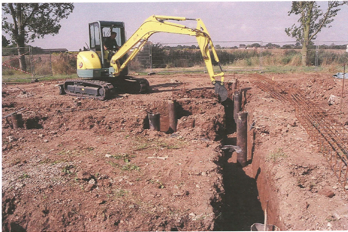
PI. 4 View of northern foundation trench looking west showing piles in situ
