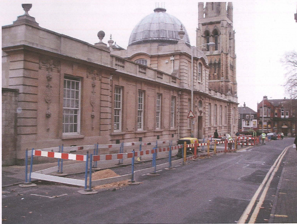
Pl. 5 View of the trench in Freeschool Lane outside the library, looking south.
