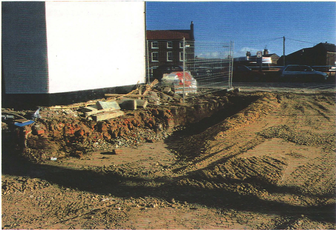
Photo. 5 Backfilled swath, excavated on north-east side of redevelopment site (largely backfilled with rubble)
