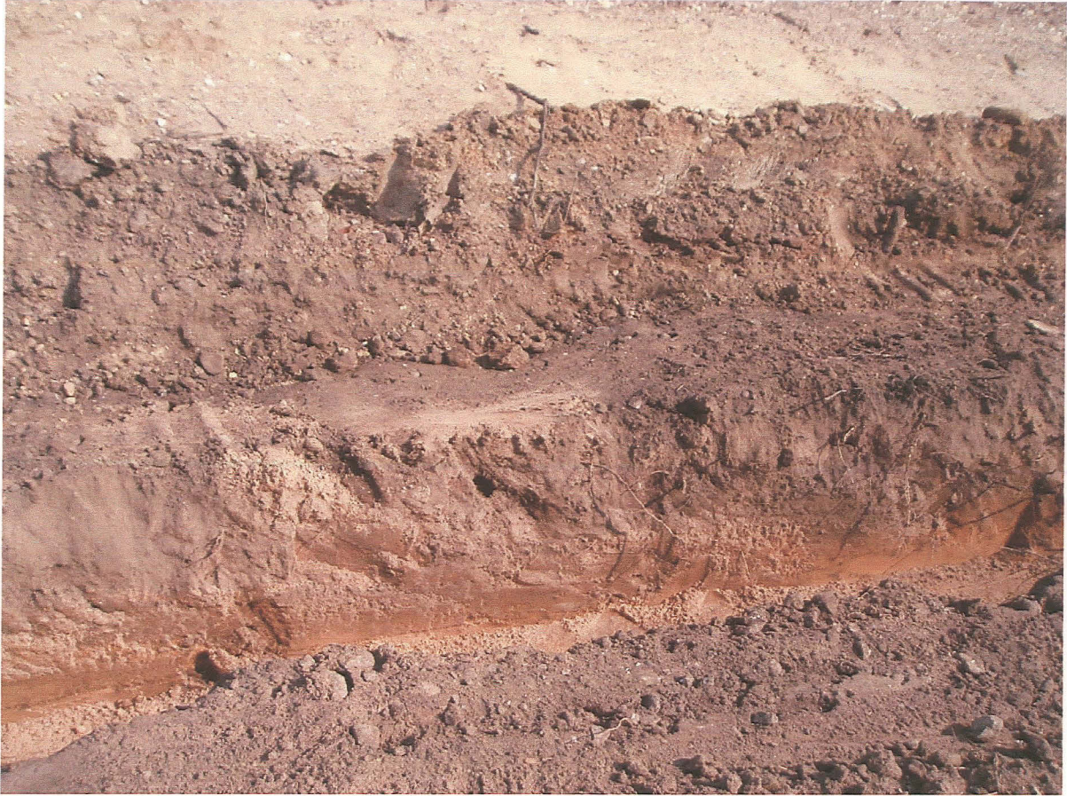
PI. 13 The detail of the northern foundation trench of the garage showing the topsoil and subsoil with the banked material above.
