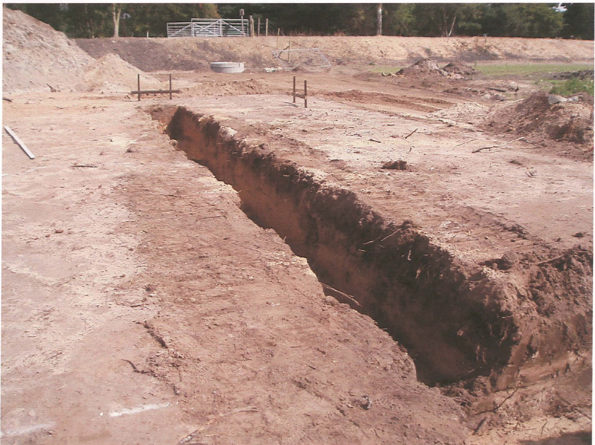
PI. 10 Detail of the foundation trench to the east of house plot 1 with the deepening of the overburden towards the south of the plot and the pond.
