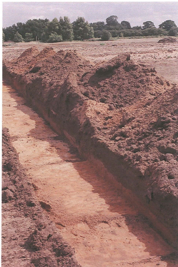
PI. 6 A section of the drains excavation trench between points D and E ( see Fig. 2).
