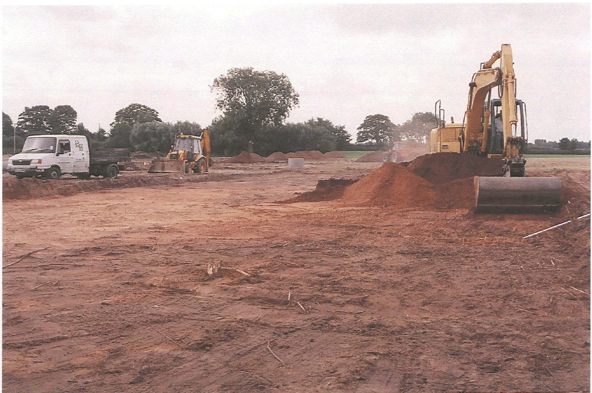
PI. 8 House plot 1 during the area stripping and prior to the machining of the foundation trenches.
