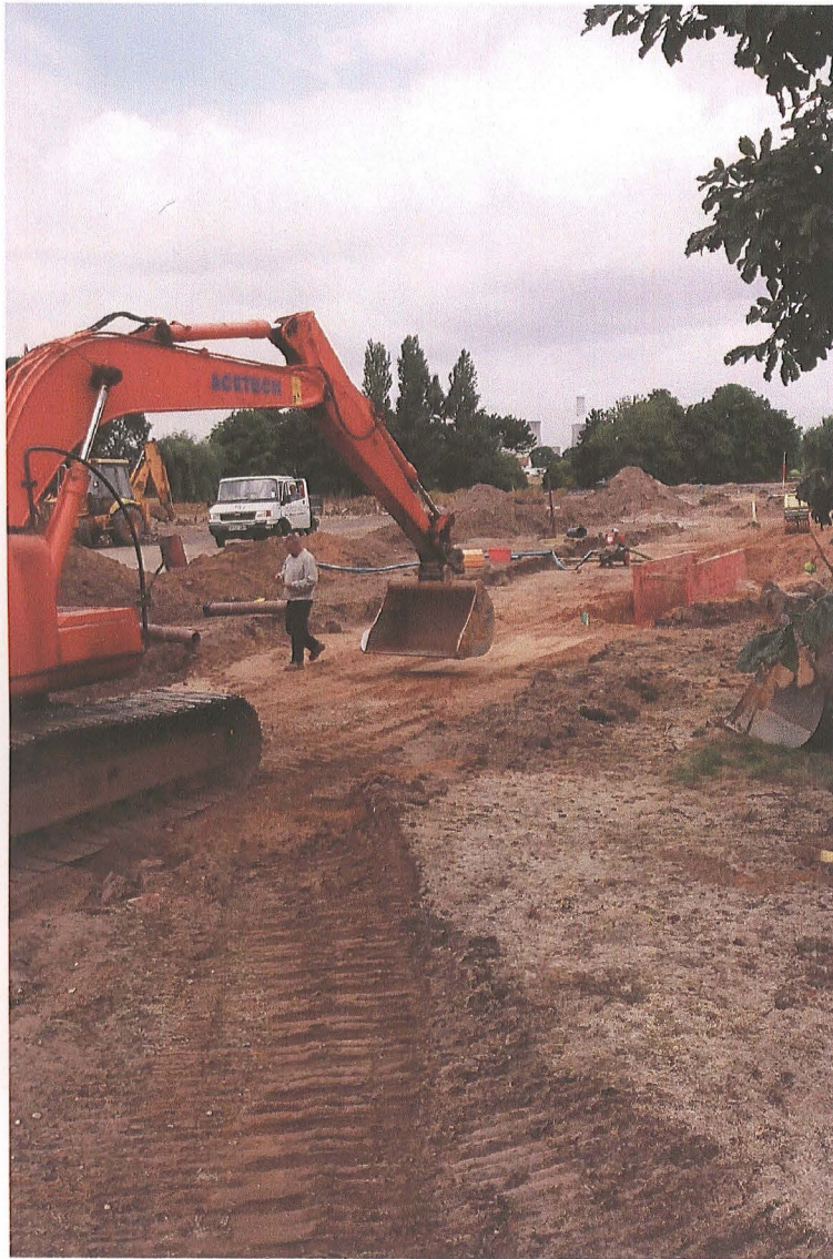
PI. 3 Stripping for the construction of the road with the steel box shoring inserted into the drainage trench.
