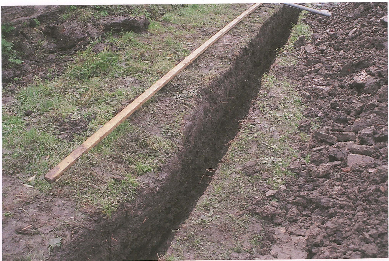
Pl. 2 Looking south along the excavated drainage trench on the southern side of the church
