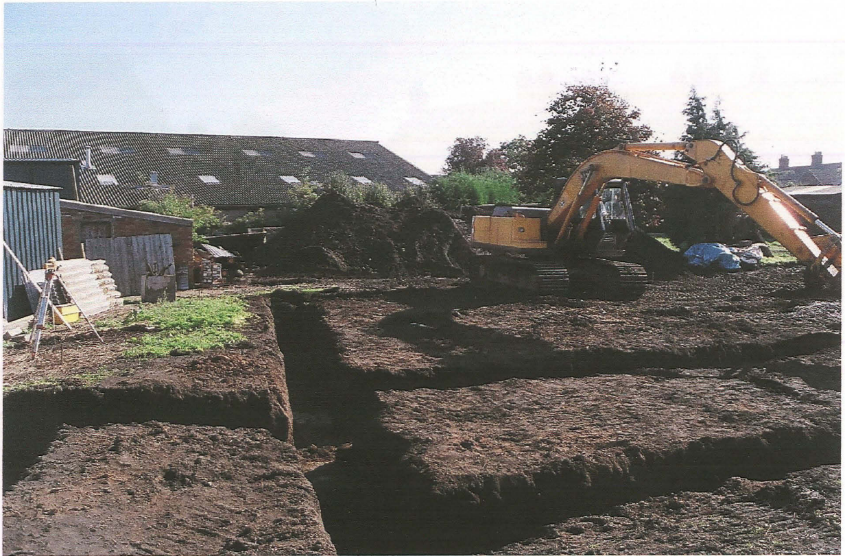
Pl. 3 Eastern half of the bungalow plot, looking south-east, with excavation in progress.
