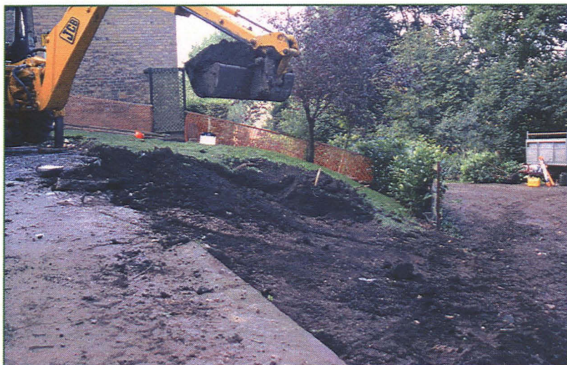
Plate 4 (left): Topsoil being stripped on the north side of the site, showing the underlying natural 002.
