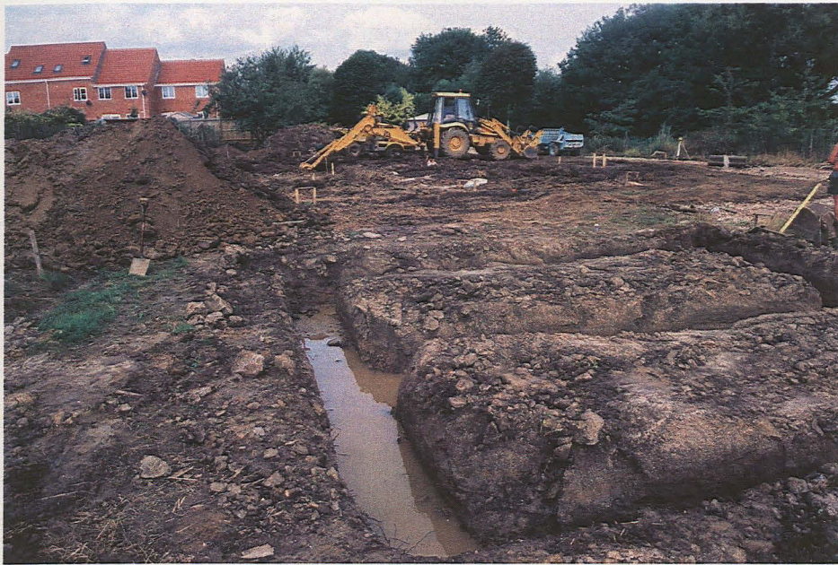
Plate 1: General view of site looking north with garage footings to the fore
