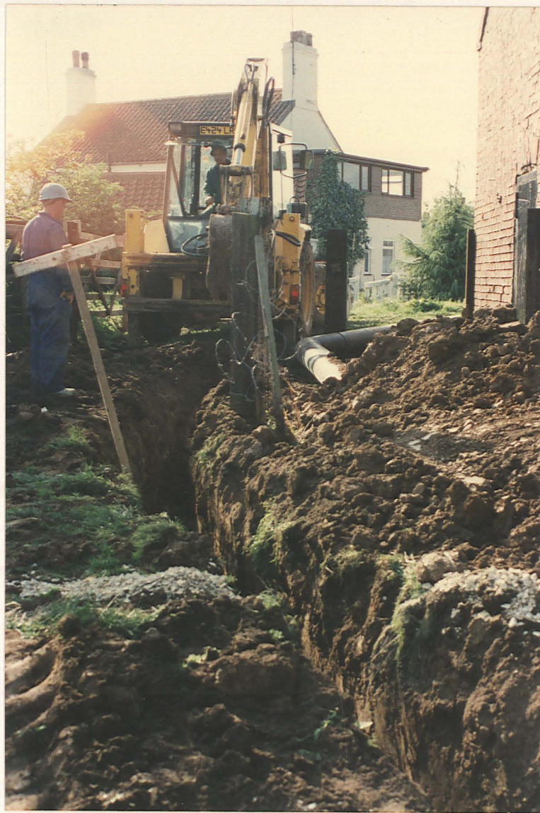
Pl. 3 Pipe trench to south of barn, Fields 1 and 2 (looking west across Catchwater Drain)
