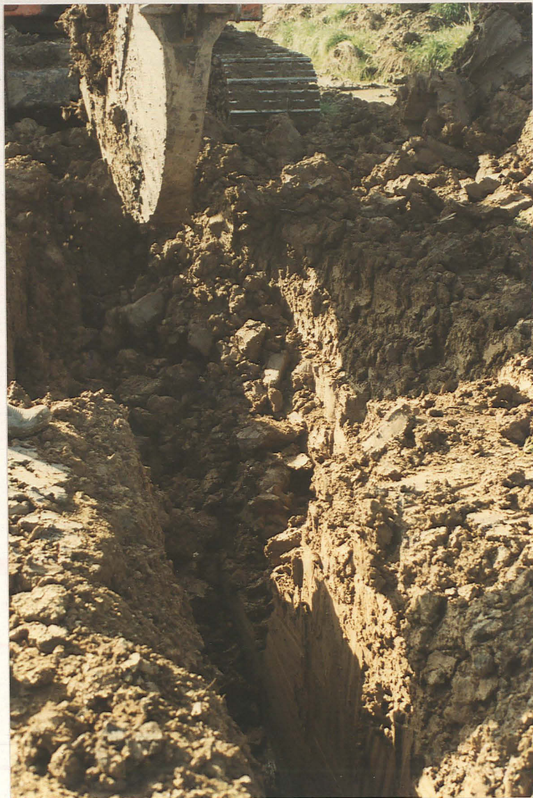
Pl. 1 Excavation of the pipe trench, using a narrow but deep-sided toothed bucket. Note the resulting smeared faces and the mixing of deposits.
