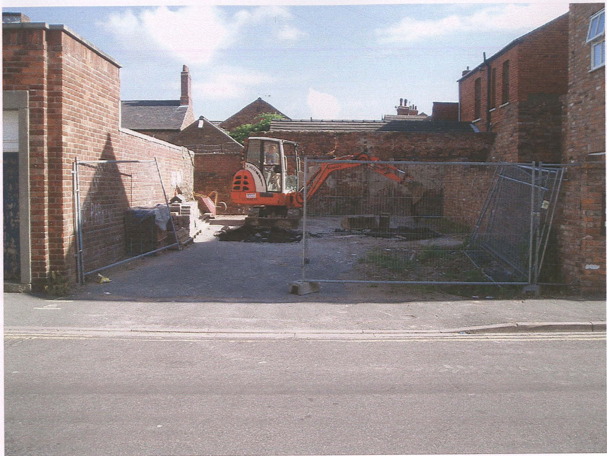
Pl. 1 General view of the site in the early machining stage. View from the south.
