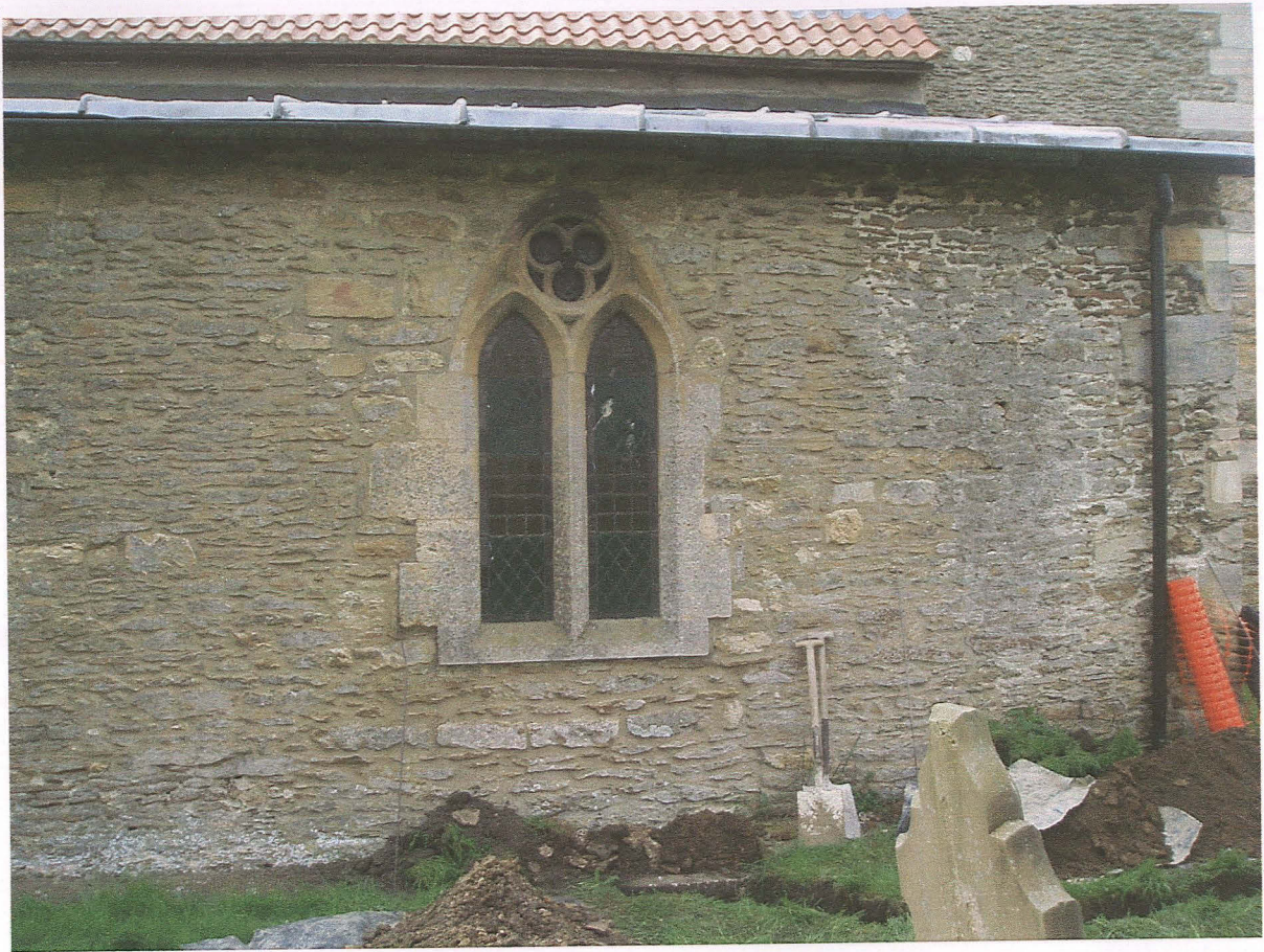
Pl. 3 The excavated pipe trench and its junction with the north aisle wall.
