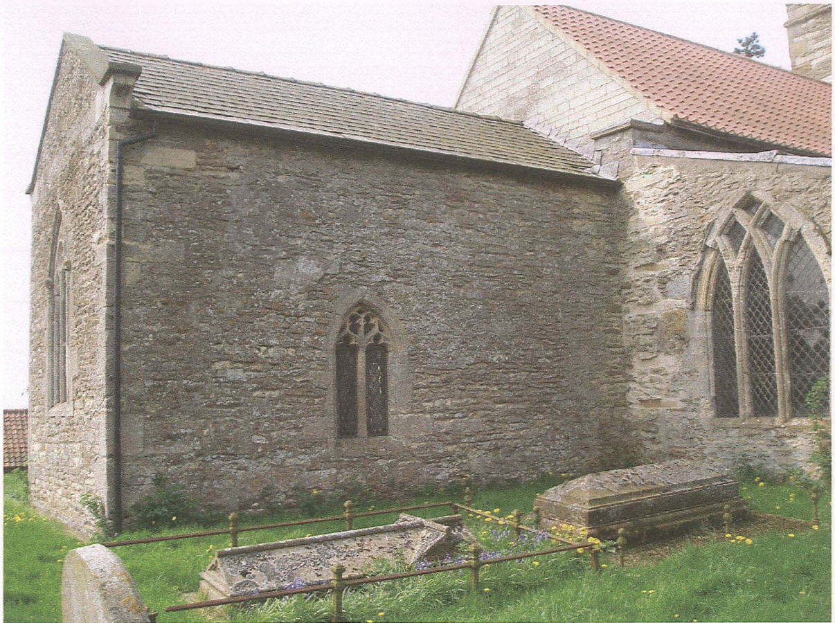
Pl. 8 The north aisle east wall showing structural cracks above the window and and recent repairs at the junction between the aisle and nave.
