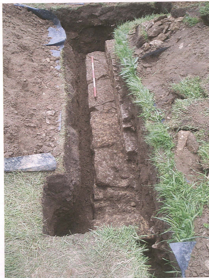
Pl. 4 The original north aisle wall within the east end of the excavated pipe trench. Scale 0.50m. looking east.
