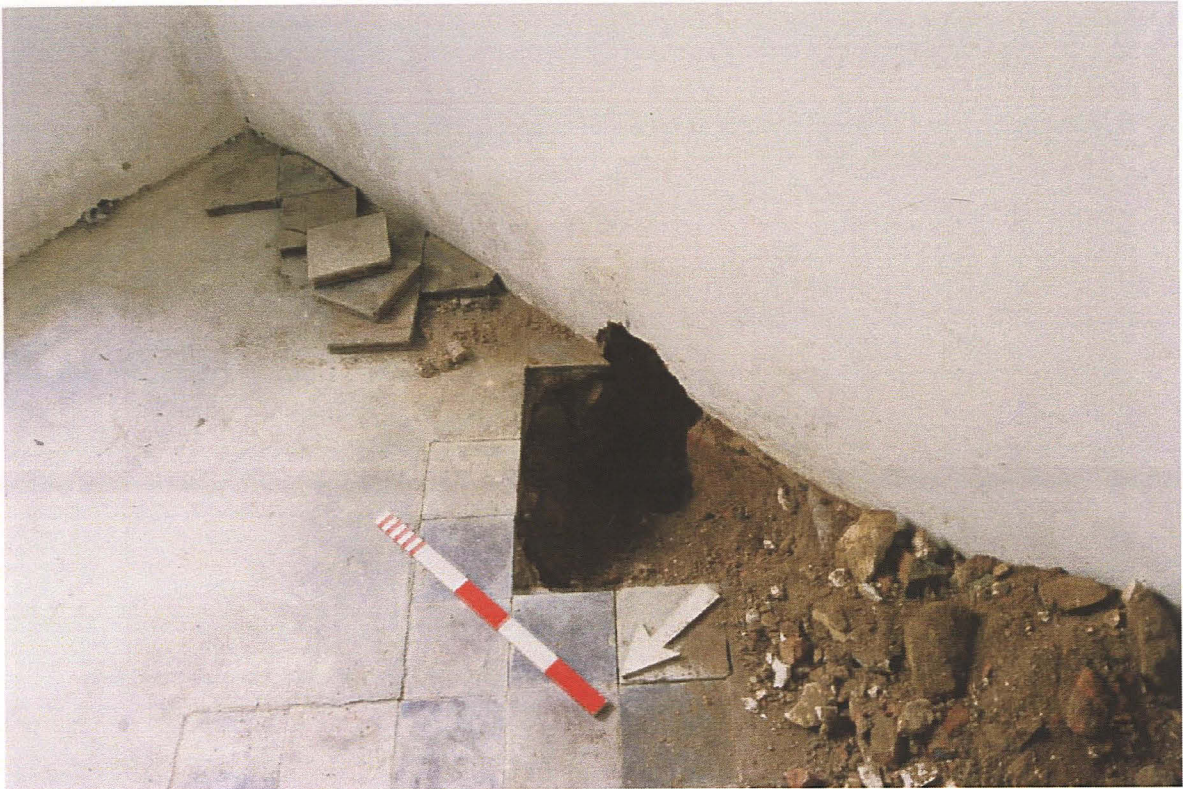
Pl. 3 Looking southeast (inside the vestry), showing the hole for the cable, drilled through the modern brick underpinning
