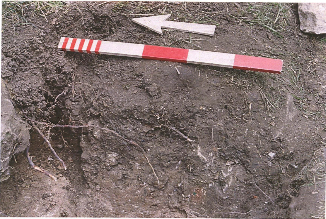
Pl. 6 Looking northeast (outside of the vestry), at the exit hole for the cable, drilled through the limestone underpinning.
