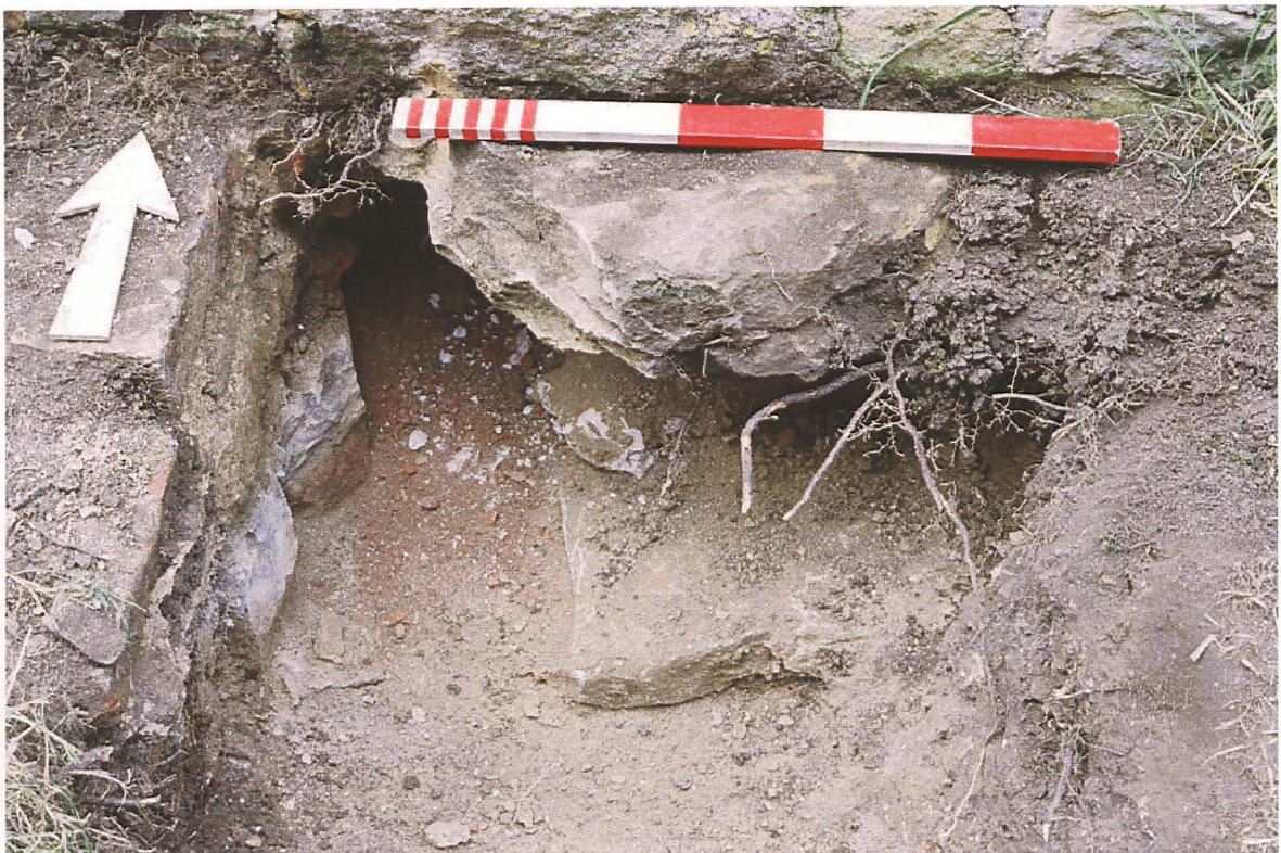
Pl. 4 Looking north (outside of the vestry), at the exit hole for the cable, drilled through (re-emplaced) limestone and brick underpinning.
