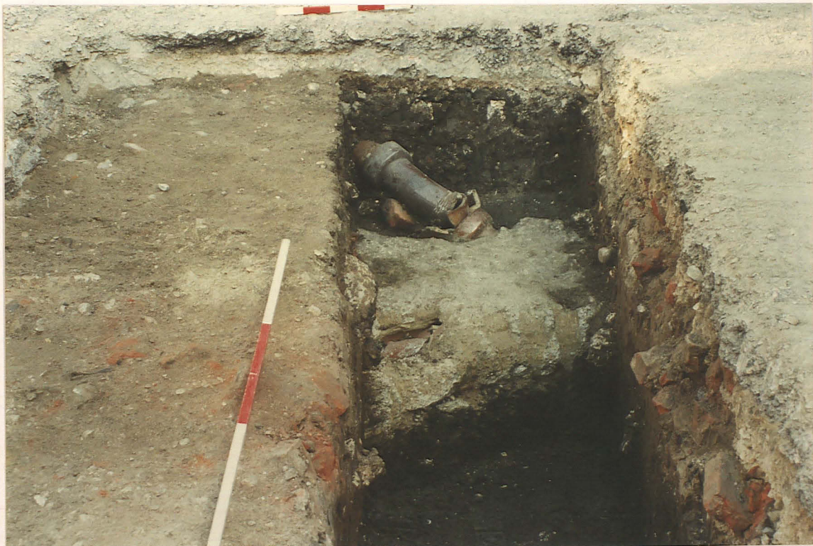
Plate 10. Trench 1. Concreted pipes at north end of trench leading to inspection chamber D (unexcavated) (Large scale 1.5m).
