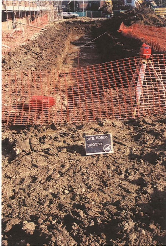
Plate 5 East facing view of culvert at eastern end of site under excavation
