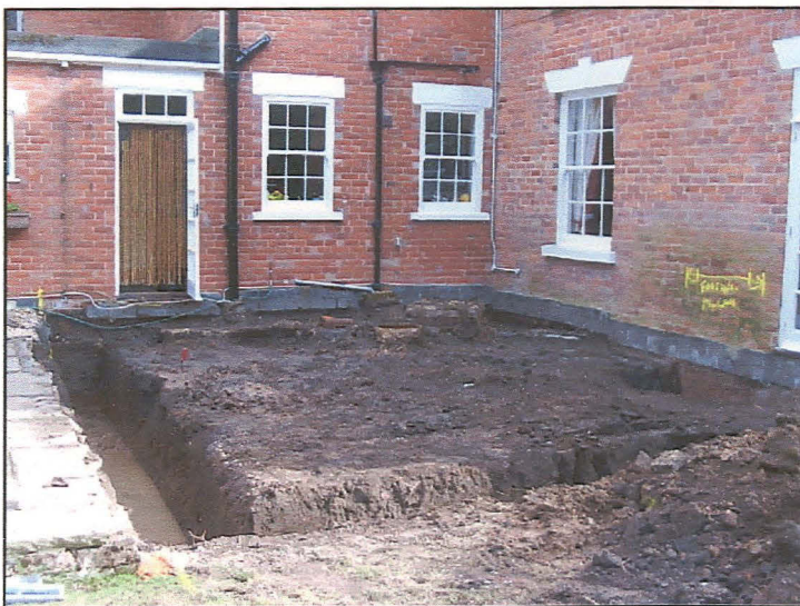
Plate 3 (left): General view of the completed footings trenches for the extension, looking south.
