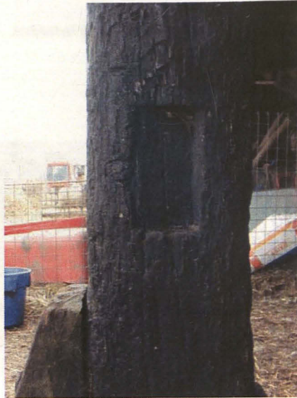
Illus 4: Upright, un-converted oak post with early (possibly Saxo-Norman) chase mortice. Note the use of large wooden dowel pegs which suggest the joint was cut before the timber was seasoned. The post is currently supporting the roof of the cart shed to the rear of No.22 High Street.
