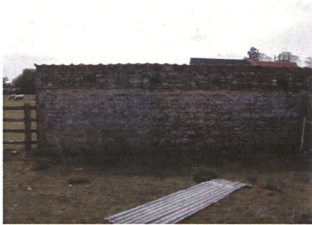
Illus 1: Southern boundary of northern pasture field. Note the surviving first floor joists within the wall.
