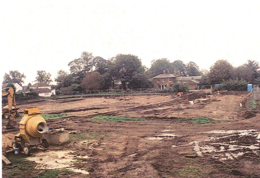
Plate 13 South facing view of site showing construction activity in progress within Area 1
