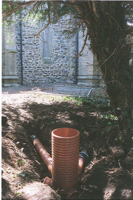
PI. 5 New drain junction north of the tower (looking south, showing rainwater pipes beside the tower).
