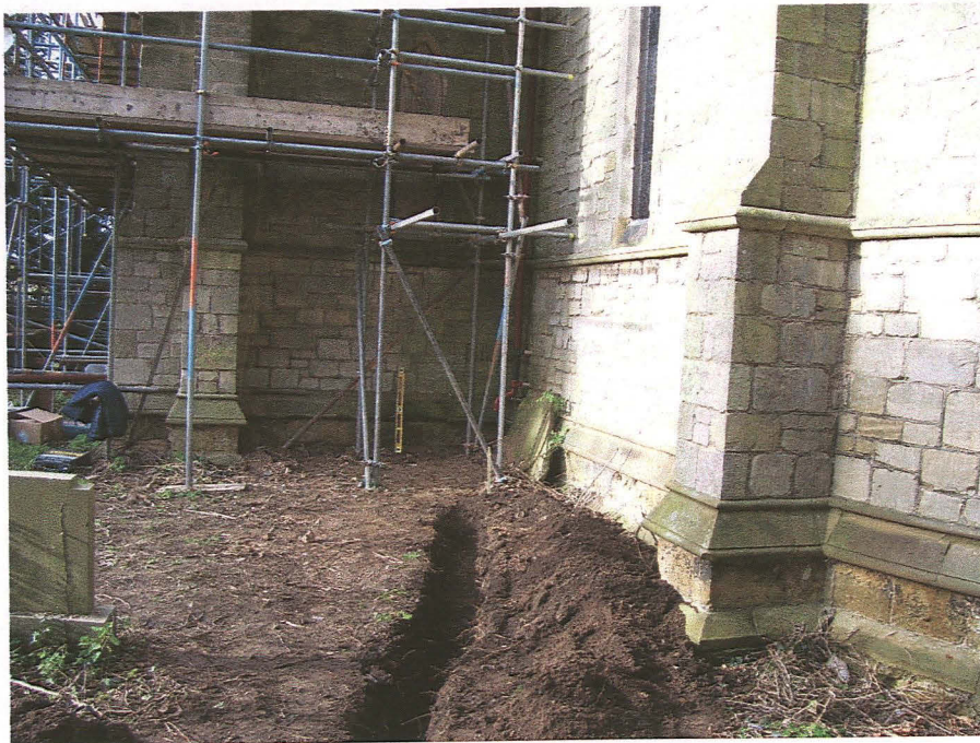
Pl. 2 Western end of the new drain trench to the south of the chancel (looking west).
