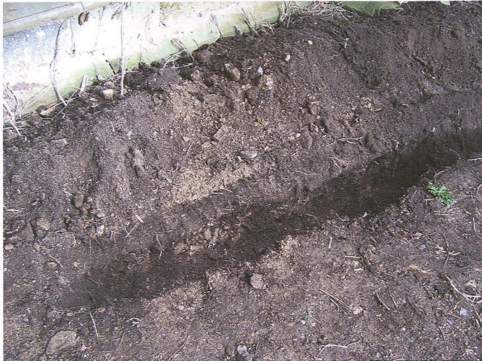
Pl. 3 Limestone chips and mortar debris in the new drain trench south of the chancel (looking north).
