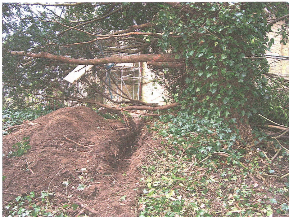
Pl. 4 Eastern end of the new drain trench to the south of the chancel (looking west).
