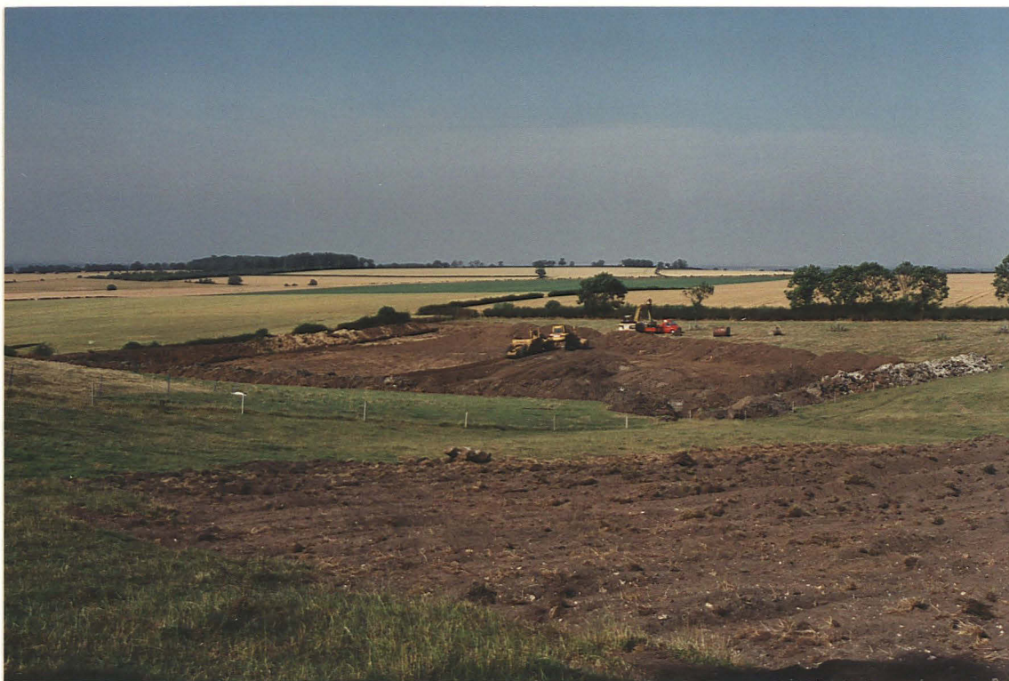
Pl. 1 Groundworks in progress for the new lake at Asgarby Hall; note the water diversion trenches on the north and south sides of the lake area. Looking SW.
