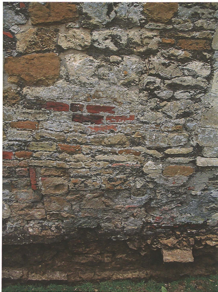
Pl. 10 Detail showing robbed out plinth course beneath area of disturbance
