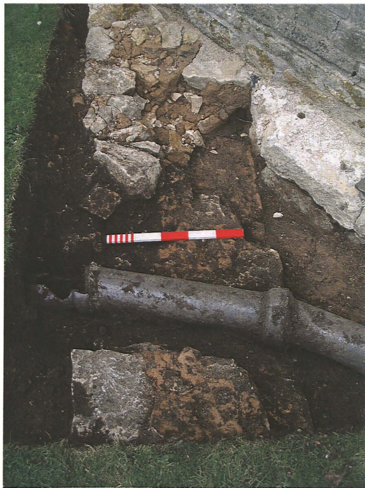
Pl. 14 Chancel south wall footings cut by drainage pipe, looking west. Scale 0.50m
