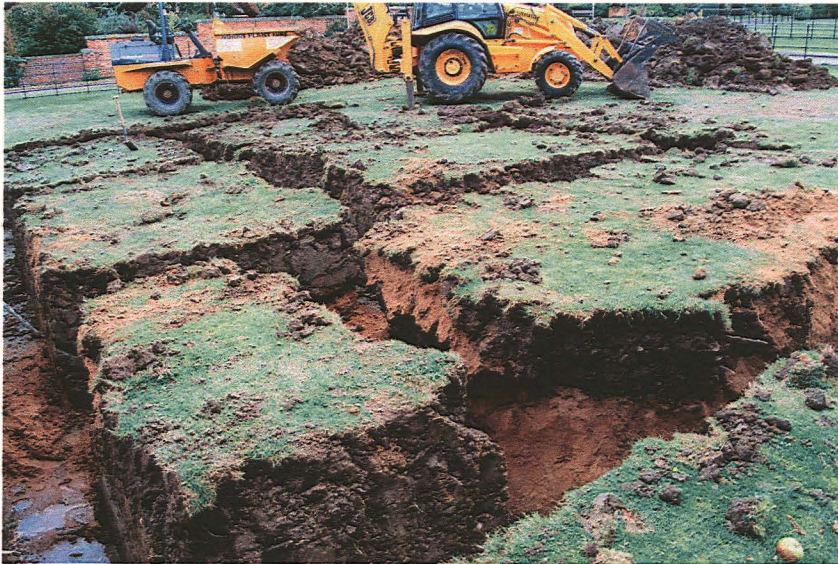
Plate 2, General view of footing trenches showing the extent of modern disturbance [003], looking east.
