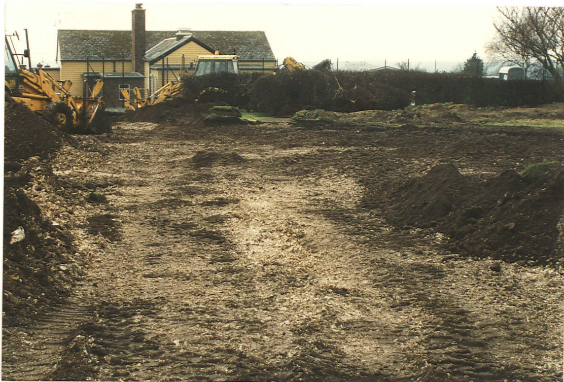
Pl. 2 Ground clearance had disturbed much of the grassed area before monitoring began, removing part of the chalk bedrock as well as topsoil and subsoil. Looking west across the Sports Hall site; a JCB is breaking asphalt in the fenced tennis court.
