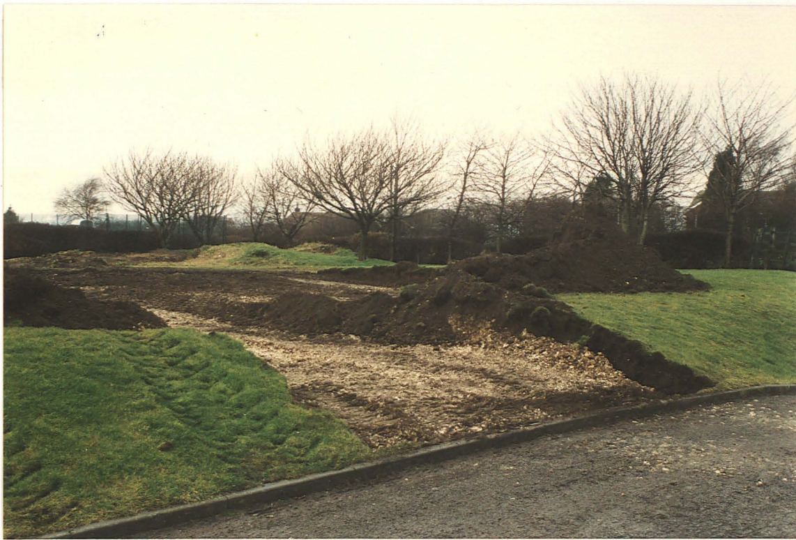
Pl. 1 Ground conditions at the start of the watching brief. The landscaped ridge can be seen in the foreground beside the school access road, with a previous spoil heap in the background close to the road hedge. The tennis court lay behind the hedge at the left of the photograph. Looking NW.
