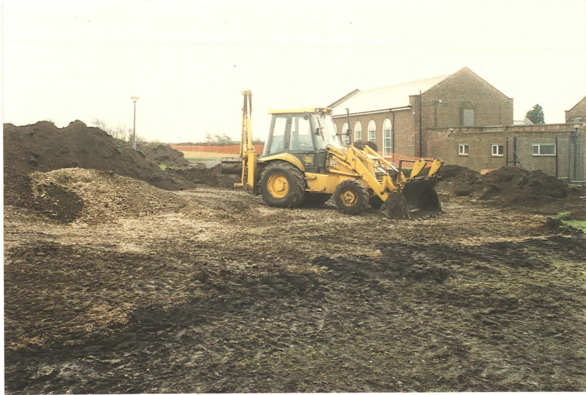
Pl. 7 Stripping of the former tennis court area revealed only previously cleared bedrock cut by a recent service trench (dark material with gravel in the foreground). Looking SE, with compound area fenced with orange plastic.
