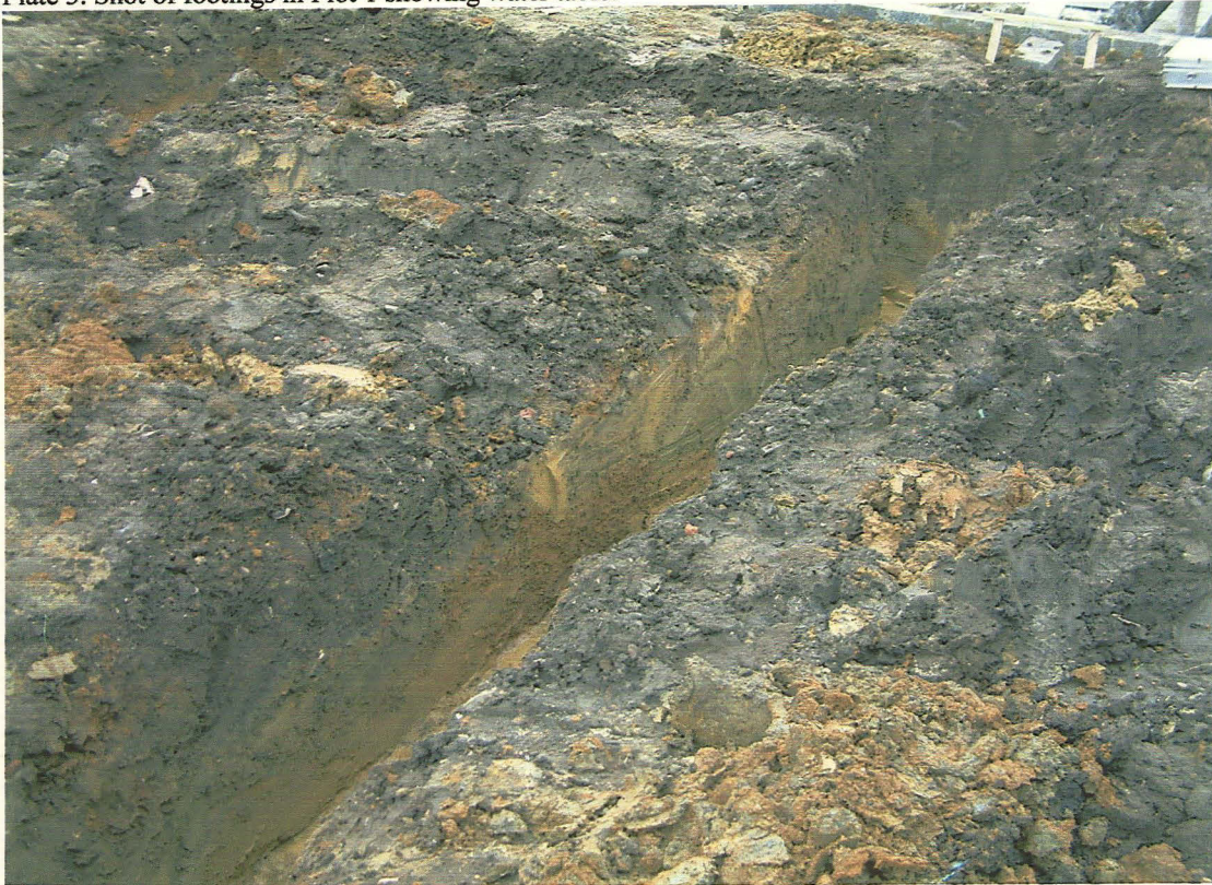
Plate 4. Showing general shot of footings in Plot 1 showing iron panning.
