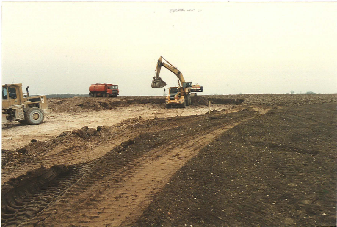
Pl. 2 Removal of topsoil and overburden to chalk within the extension area (looking south)
