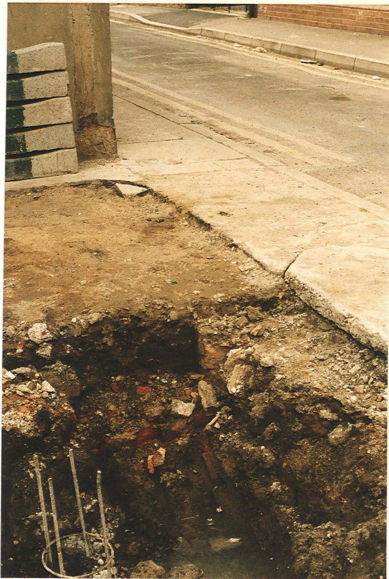
Pl. 3 Hole beside Pile 12, showing brick wall foundation and level of standing water (looking east onto Union Street)
