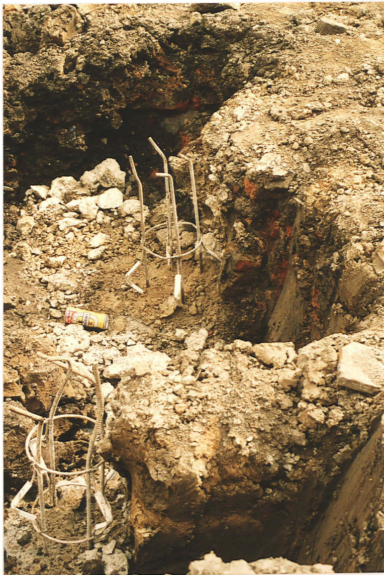
Pl. 2 Holes dug around Piles 14 and 18, revealing brick walls of cess pit or cellar
