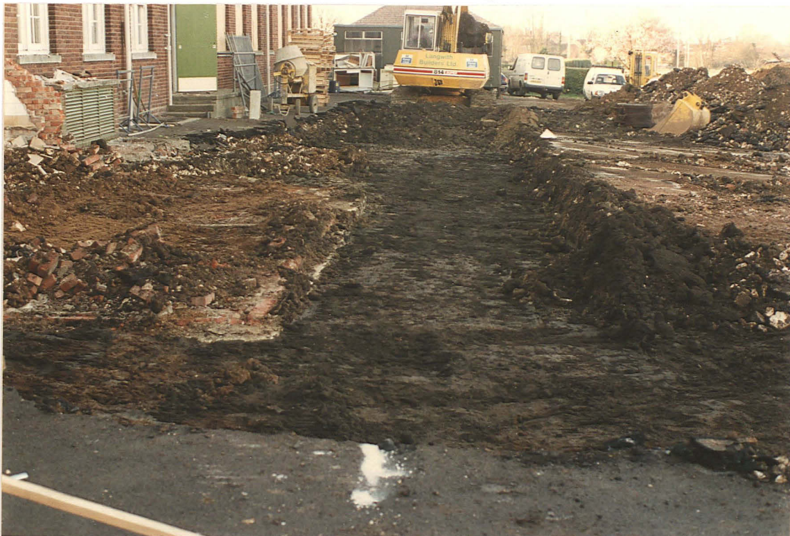
Pl. 4 Foundations of demolished changing rooms. The dark fill of Pit 10 is visible in the foreground, with undisturbed orange subsoil to the left of the white chalk mark. Looking NW.
