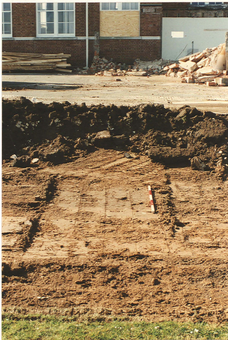
Pl. 3 Surface of subsoil after removal of turf and topsoil; looking west to the school building with the tarmac playground on chalk rubble and buried topsoil. Scale divisions 0.2m).
