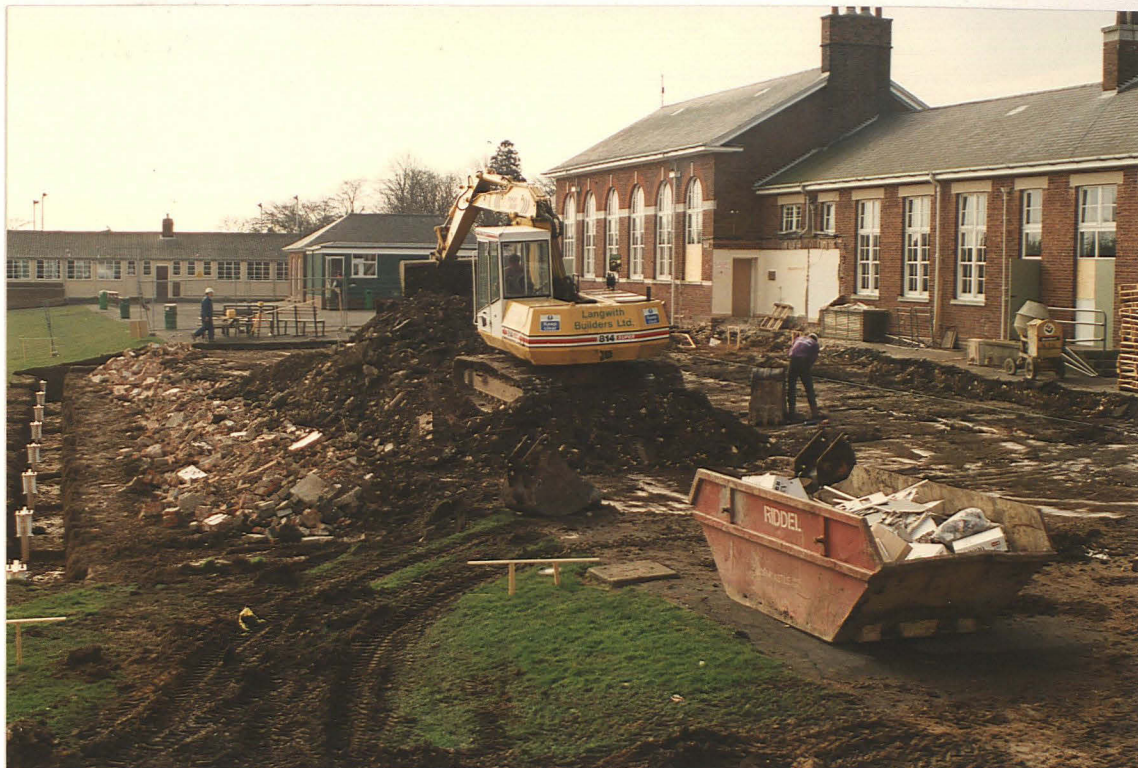
Pl. 1 Groundworks in progress at Sir John Spendluffe School. Modern brick rubble has been used to raise the ground in place of a former slope. Looking south.
