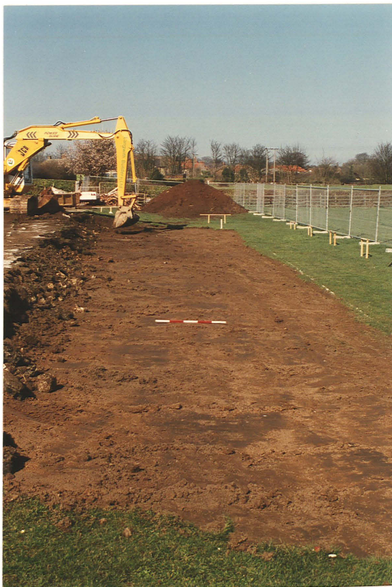
Pl. 2 The turf and topsoil slope was removed before trenching began. (Looking north; scale divisions 0.2m).
