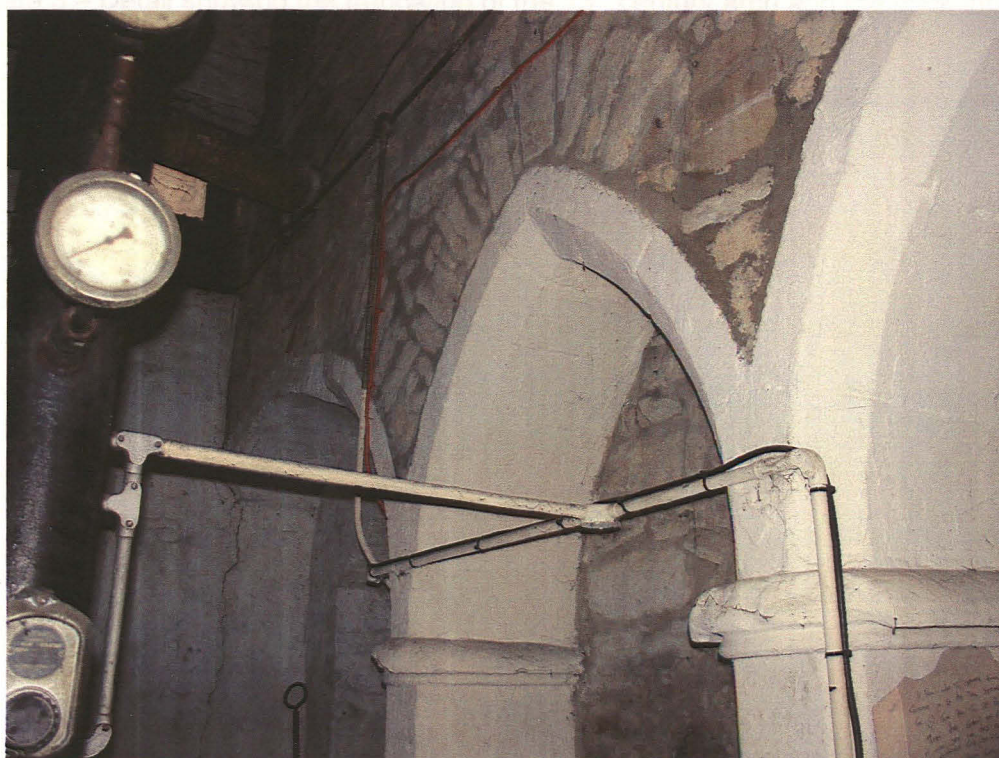
Plate 2 – View showing the blind arcade within the boiler room. The proposed new passage is to be located in the furthest arch
