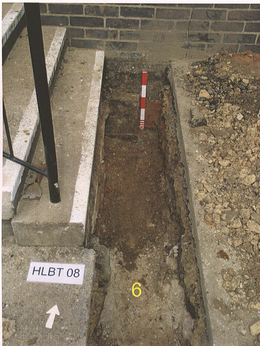
Pl. 4 North end of trench, showing stair foundation 6 looking north. 1 x 0.5m scale.
