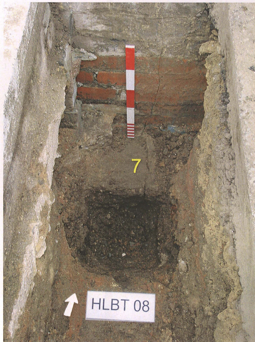
Pl. 5 Detail of Library foundation 7. Note structural crack and investigative slot to establish base of foundations, looking north.
