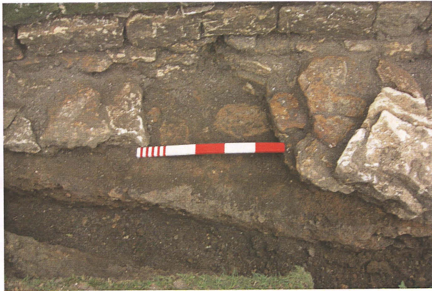
Pl. 19 Damaged area of tower north foundations, after removal of infill soil, scale 0.50m
