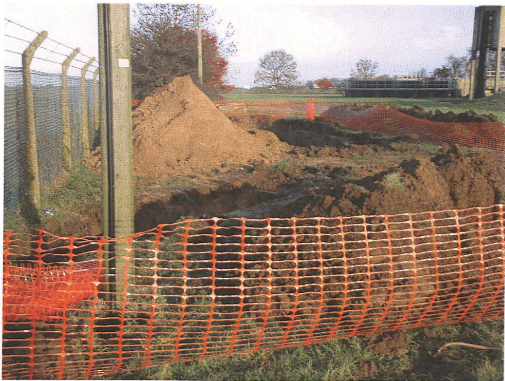
PI. 6 Location of Pits 11 and 12 within the sewage works compound (looking north).
