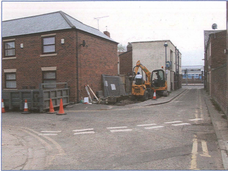
Plate 1: General view of the site during the groundworks, looking east from Mill Lane.
