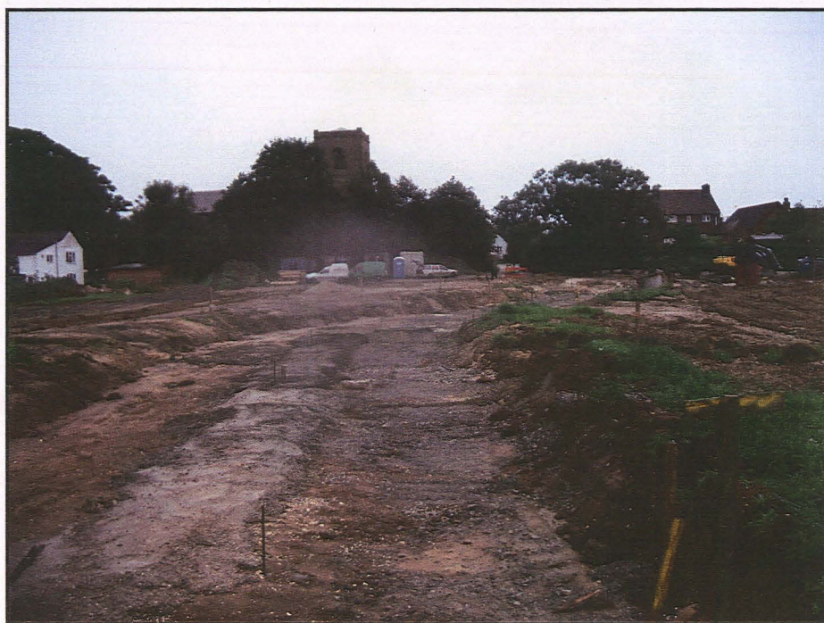
Plate 1: General view of site looking south showing a section of the unmonitored road strip and concreted sewer trench
