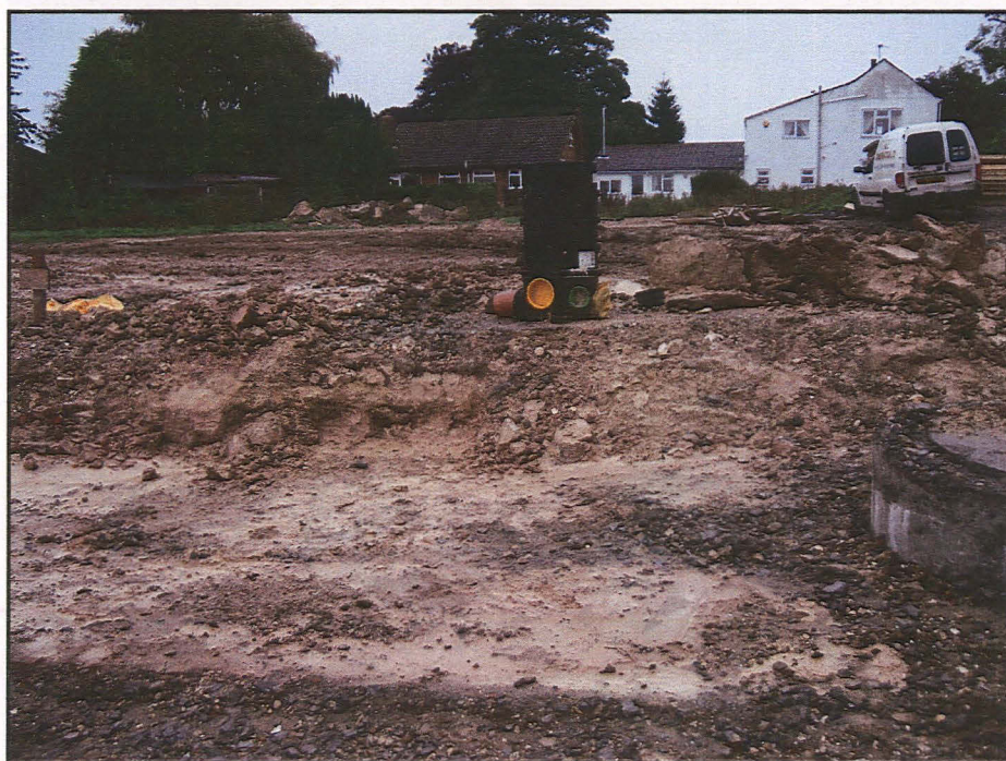
Plate 2: General view of the site looking east also showing part of the road strip
