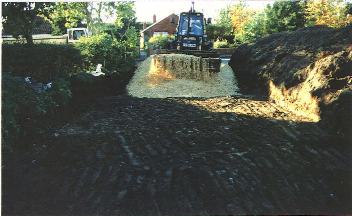
P1. General view of area west of building plot after excavation and during infilling of site access/parking area; looking west towards Church Street
