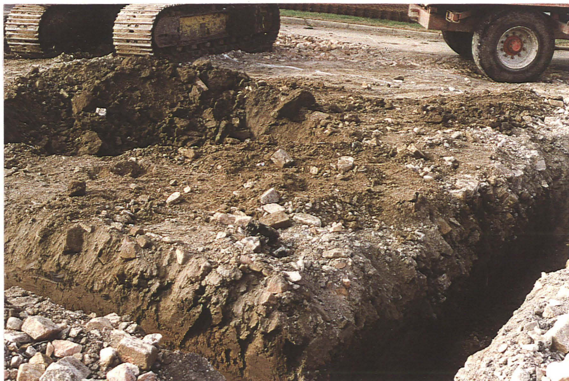
Pl. 6 Location of hole dug by the contractor to bury concrete lump, between the northern and central excavated trenches. (Looking SW).
