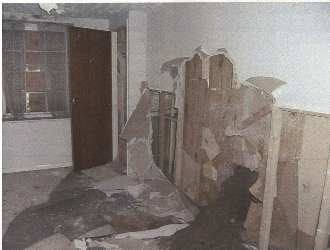
Plate 23 Interior of Room 1a, showing recesses and fireplace behind stud partition wall, looking southeast
