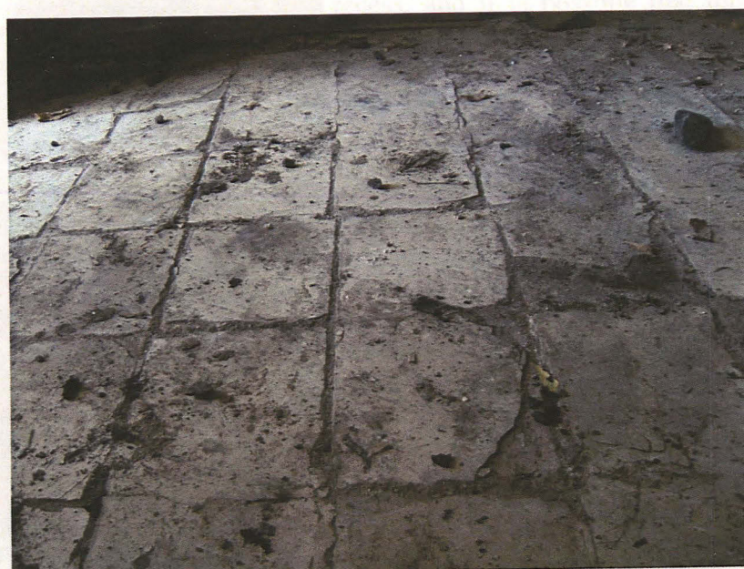
Plate 57 Interior of Room 2a, detail of flooring of concrete, apparently poured over ceramic tiles, looking north
