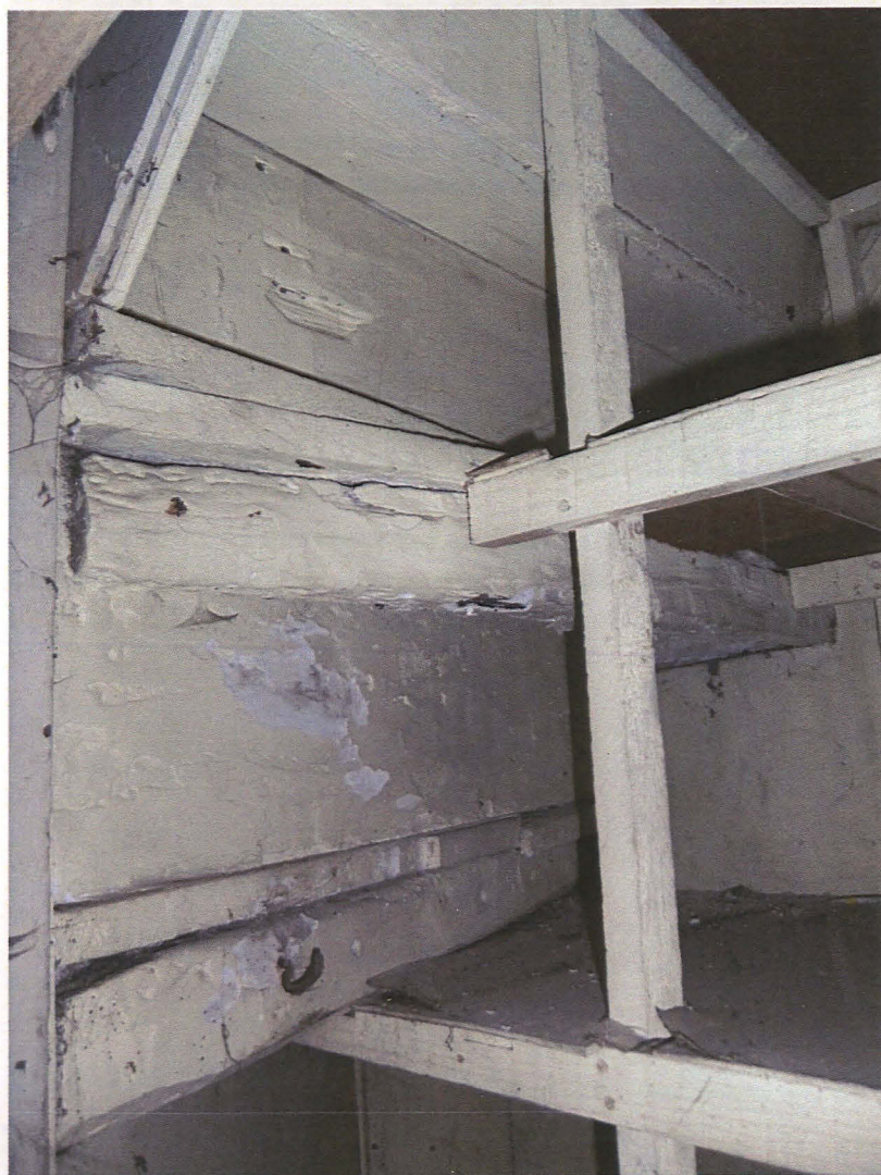
Plate 29 Interior of Room 1a, detail of underside of staircase and shelving in alcove behind stud partition wall, looking southeast
