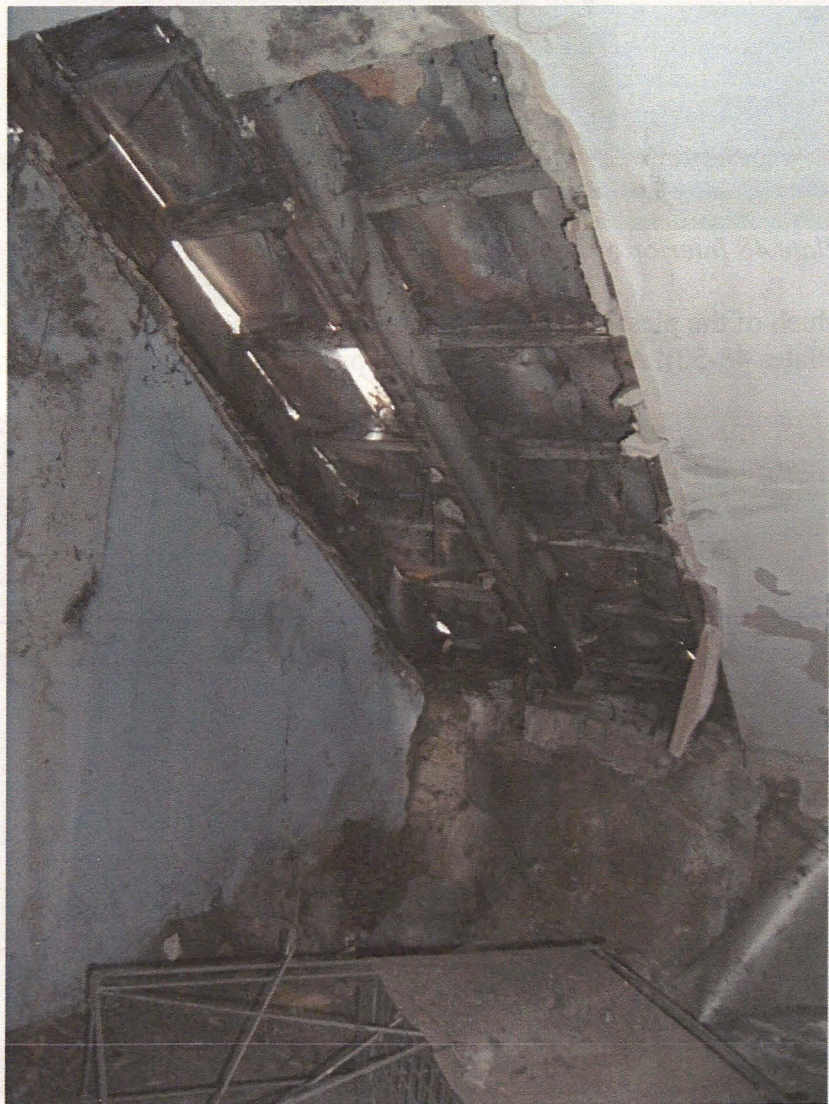
Plate 51 interior of Room 2b, showing roof structure with pantiles and hole in corner of floor, looking southwest
