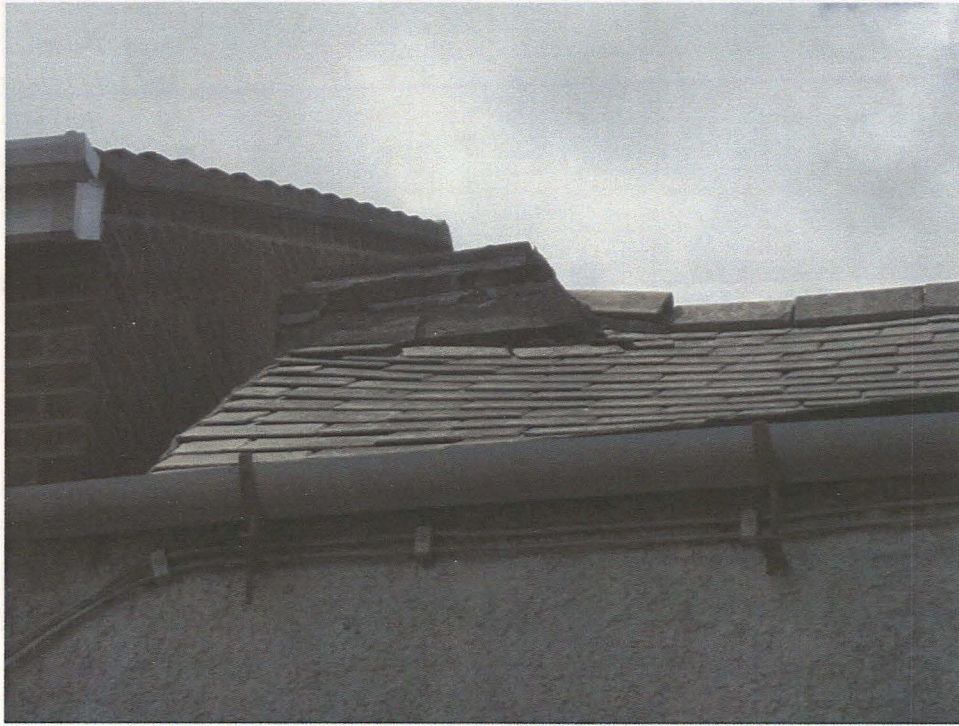
Plate 13 Detail of remnants of recently- removed chimney at south gable end of building, looking west
