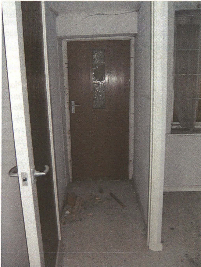
Plate 21 Interior of Room 1a, detail of doorway and stud partition porch, looking east
