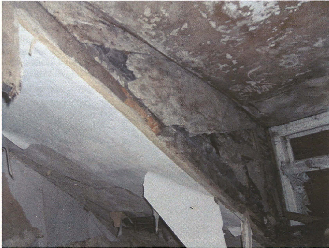
Plate 39 Interior of Room 1b, detail of construction at north cheek of dormer window, looking northeast
