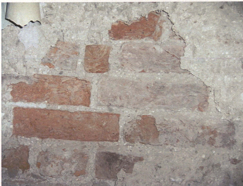
Plate 44 Interior of Room 1b, detail of exposed brickwork of south wall, looking south
