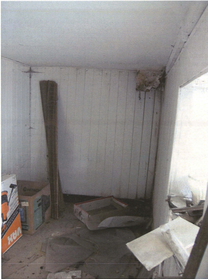
Plate 53 Interior of Room 2A, showing wood panelling, window and hole in corner of ceiling, looking south
