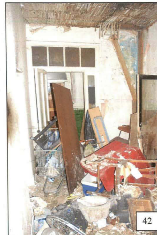
Plate 43: 47, St Catherines – Room 9, first floor fire damage.
