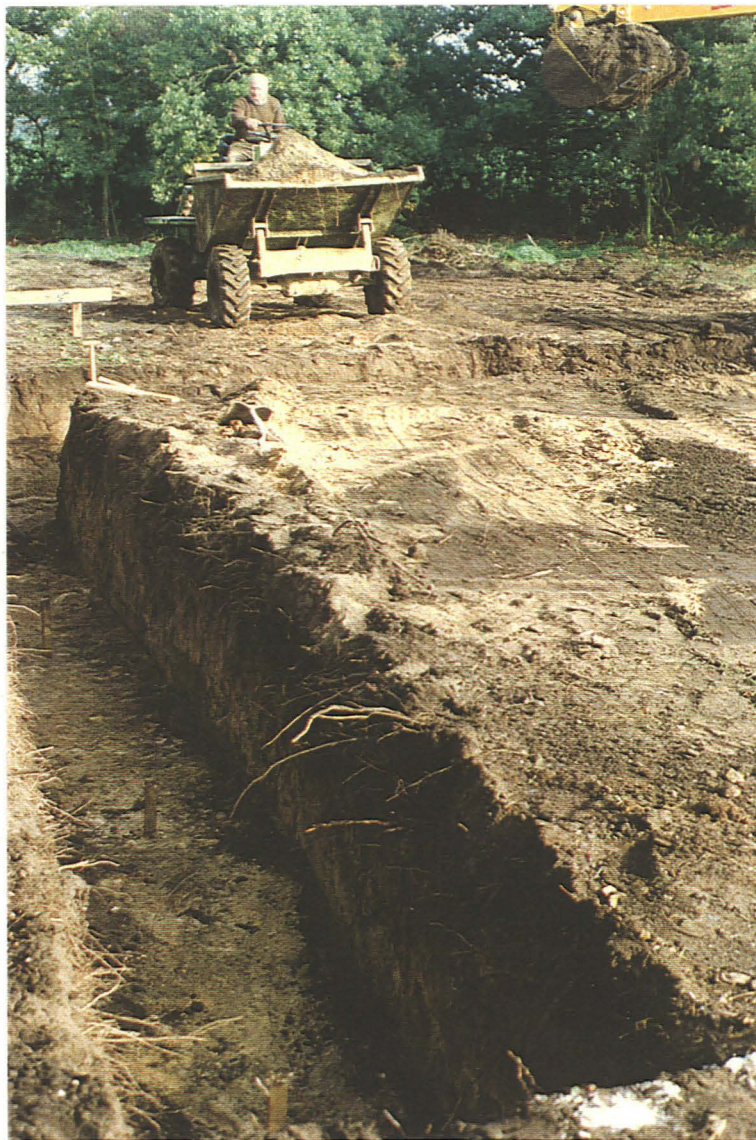
Pl. 6 East face of the western foundation trench; Ditch 1 crosses beneath the shovel (looking north).
