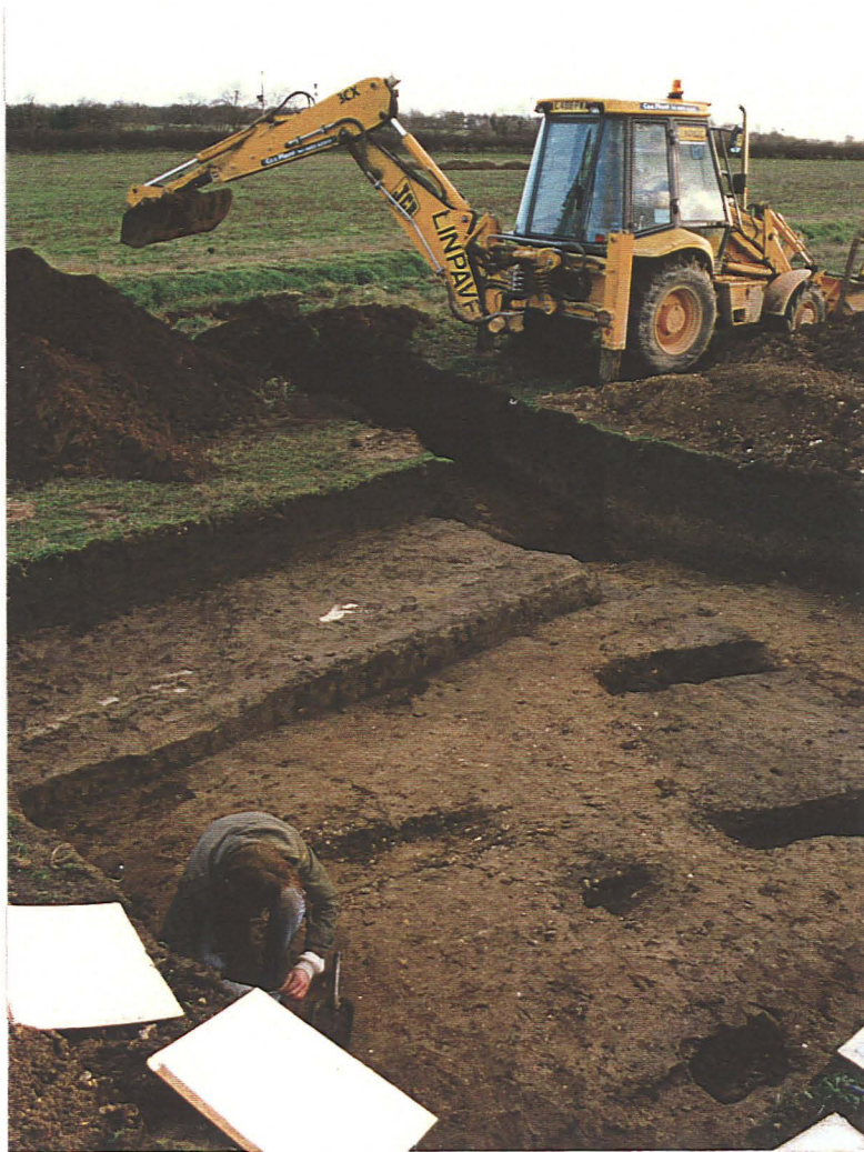
Pl. 16 Trench 20, extending trench to south-east; remainder of stiff clay lens 158 being exposed in section. Looking south.
