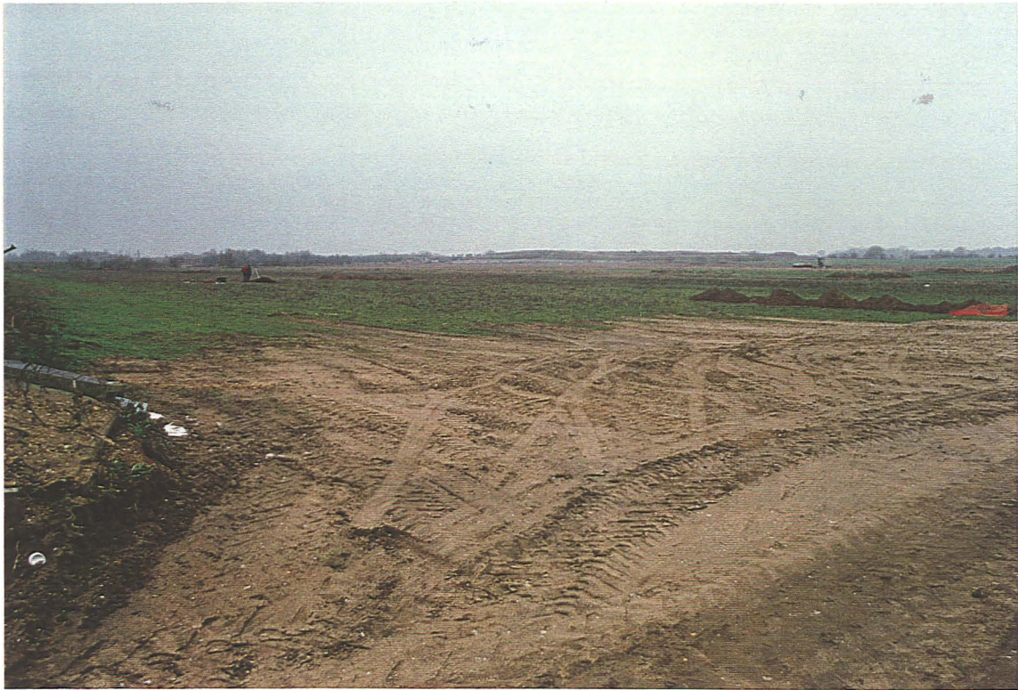
Pl. 20 General view from site entrance, looking west. Sieving in progress in Trench 27 (left part of picture).
