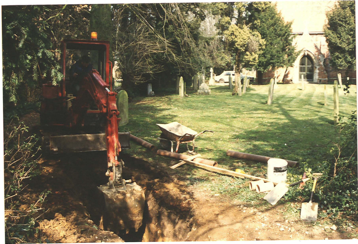
Pl. 1 Trenching in St. Peter's graveyard; the path curves behind the mini-excavator towards the car (looking NW).
