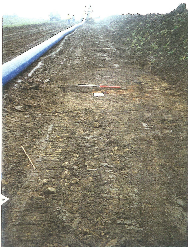
Plate 1. General View along the pipe line easement. Section 1 lies in the foreground.
