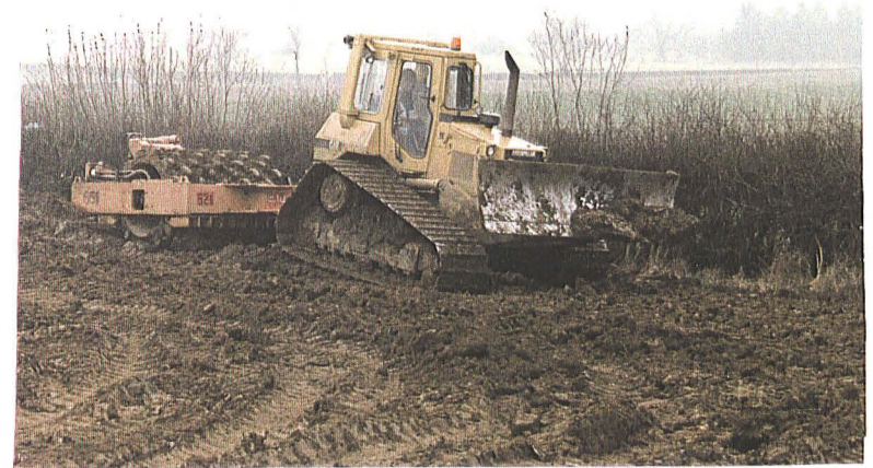
P2- Bulldozer battering down lias clay core of Flood Bank 1, looking south
