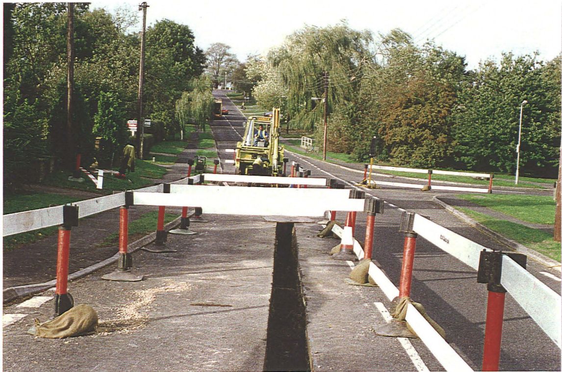
Pl. 14 Location of 4, marked by the excavator close to Kingsway (looking west towards the A46).
