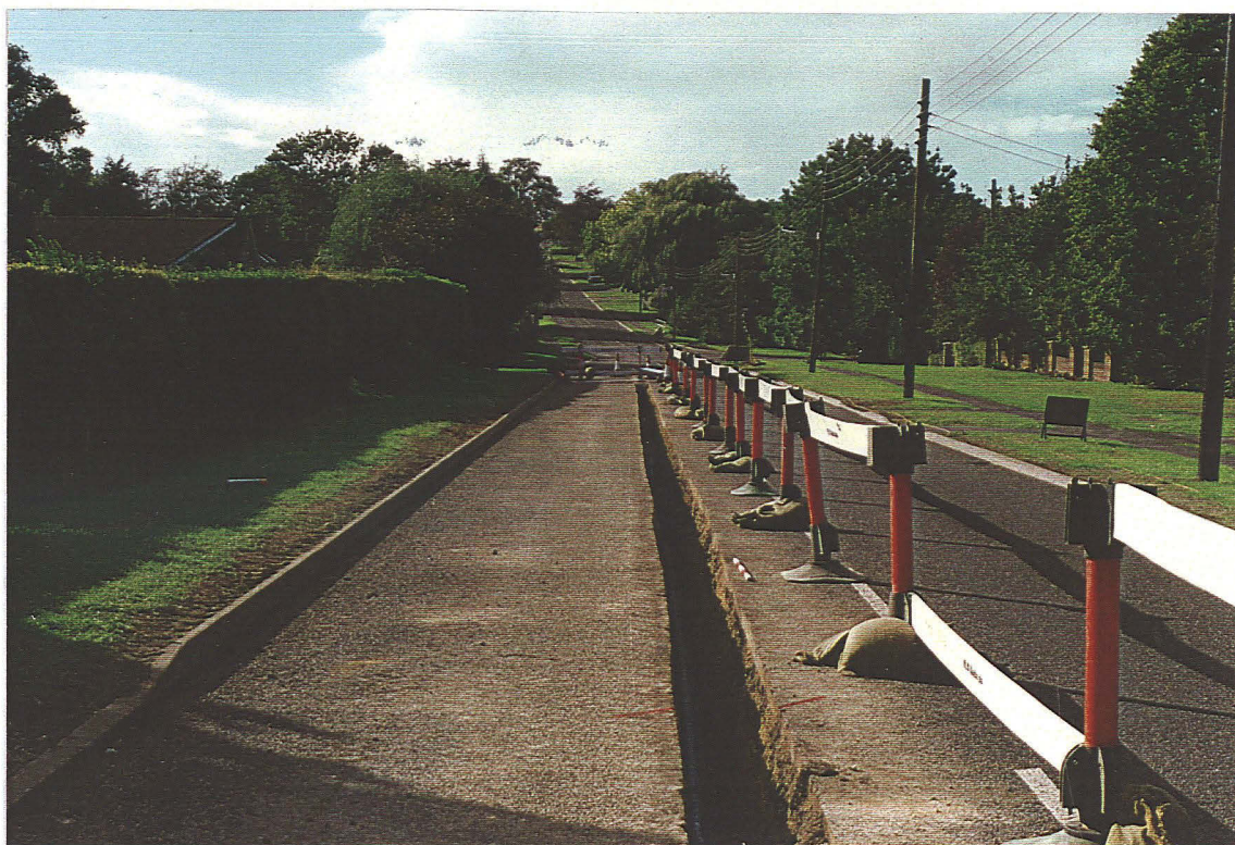
Pl. 4 The pipe trench on Washdyke Hill. The 1m photographic scale marks the centre of backfilled feature 1, probably a limestone quarry pit. The eastern edge is marked by red paint in the foreground (looking west).
