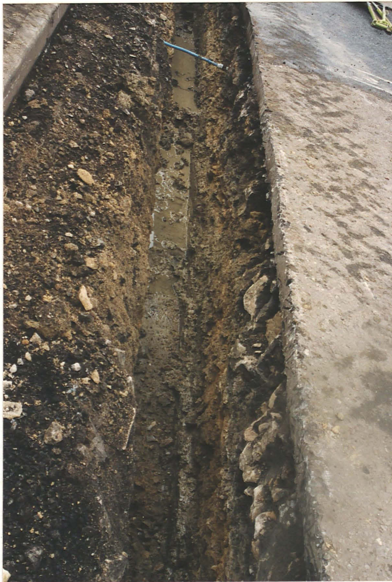
Pl. 19 Clay visible at the trench base at 5, beneath the road foundation of large stone lumps and redeposited limestone brash.
