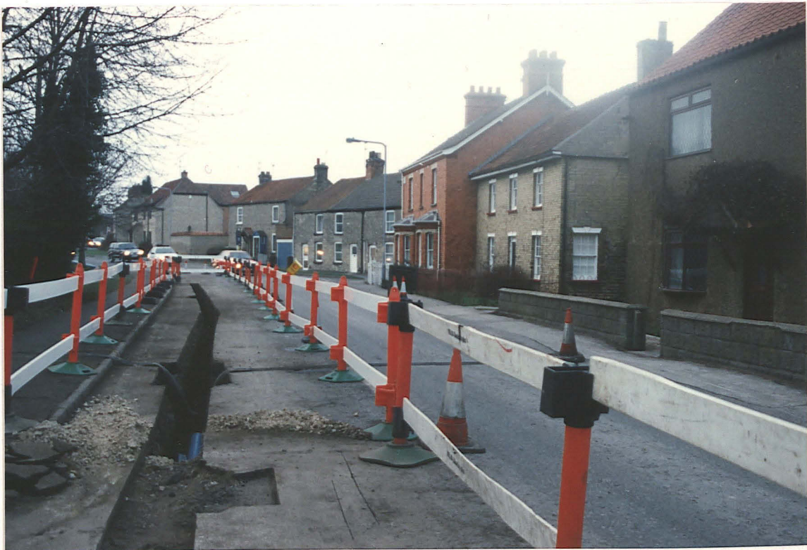
PI. 17 The pipe trench in High Street, north of the Old Bishop's Palace site (looking west).
