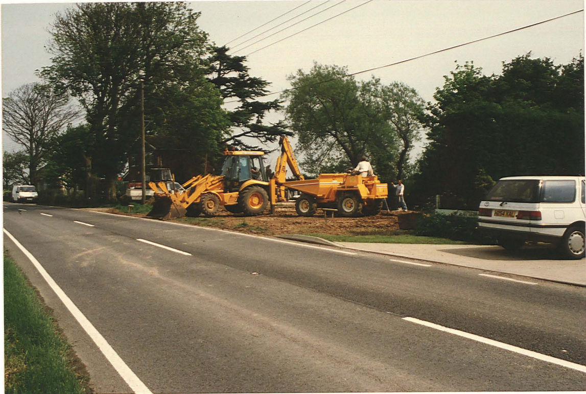
PI .1 General view of site from Sutton Road, Priory House to left.
