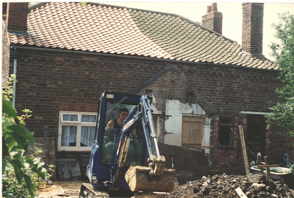
Pl. 1 Site of the new foundation trenches at the rear of Churchview (looking SW)
