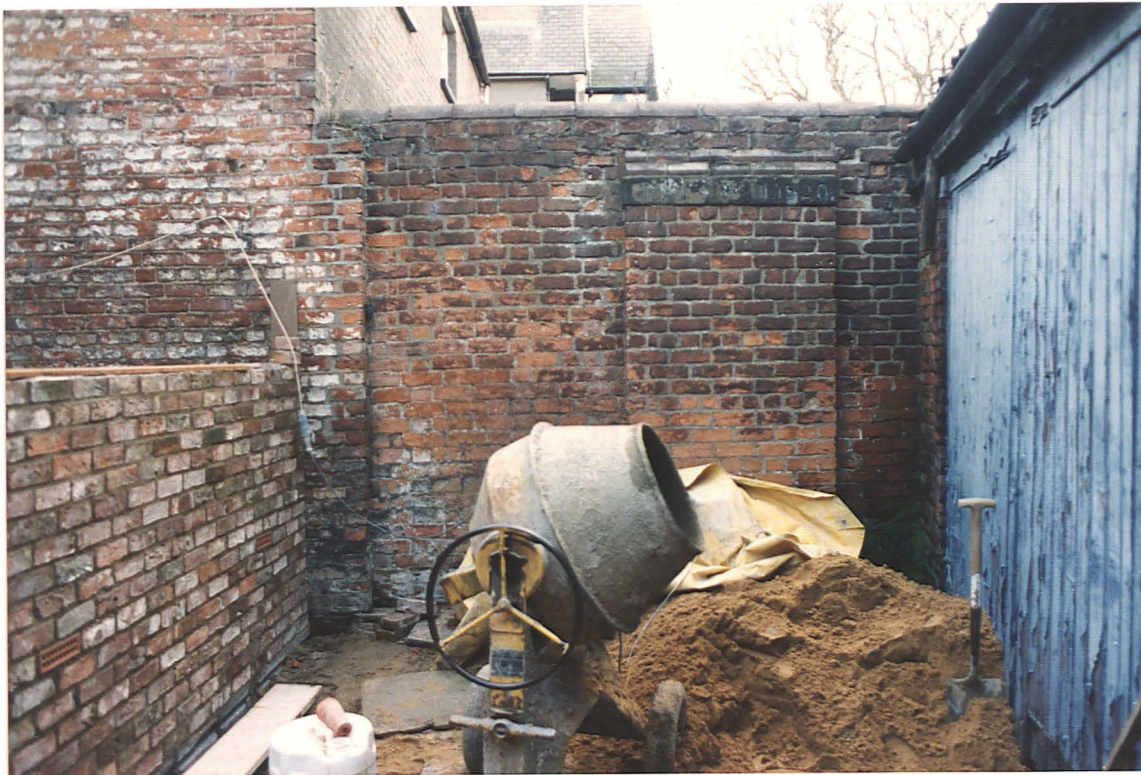
PI.8 General view of existing NE-facing wall elevation with 19th century name plate, looking SW.
