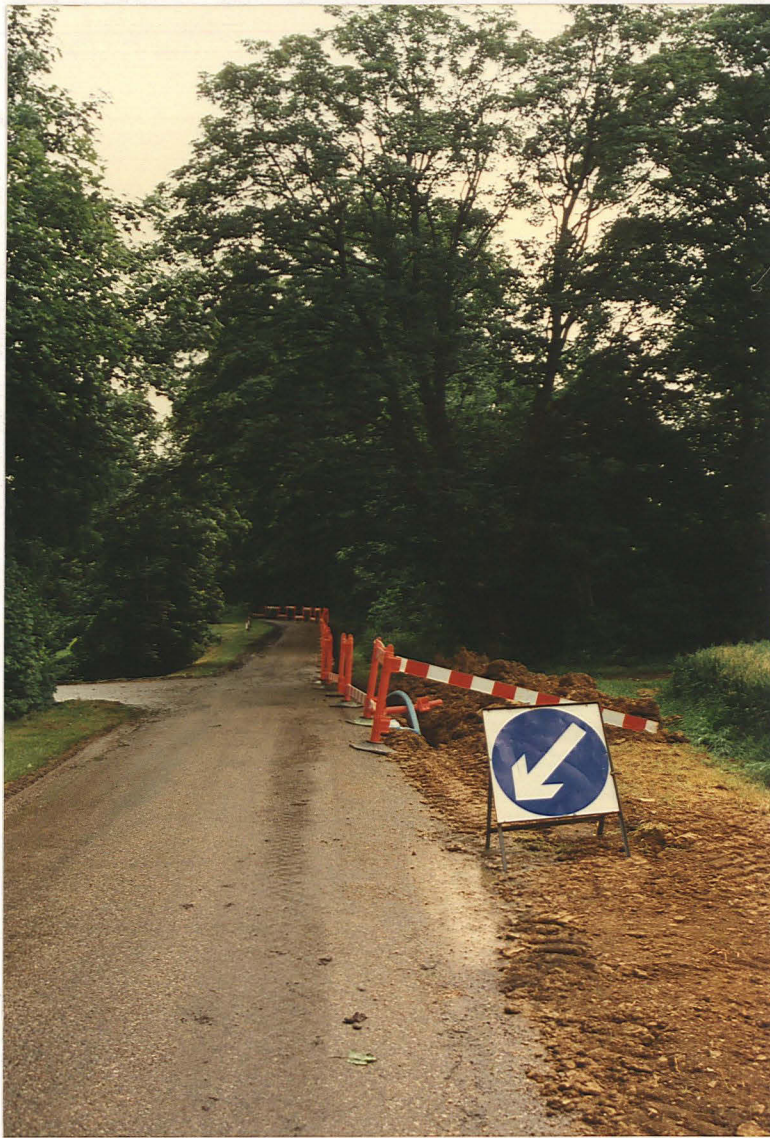
PI. 7 Springwell Plantation (to right) with pipe trench approaching stream. Looking south.
