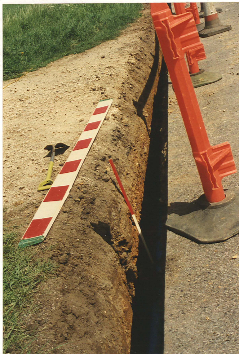
Pl. 4 View of the pipe trench cutting across the track at 6, north of the Ashy-Digby road (looking east). Scale divisions (h) 0.25m, v 0.5m.
