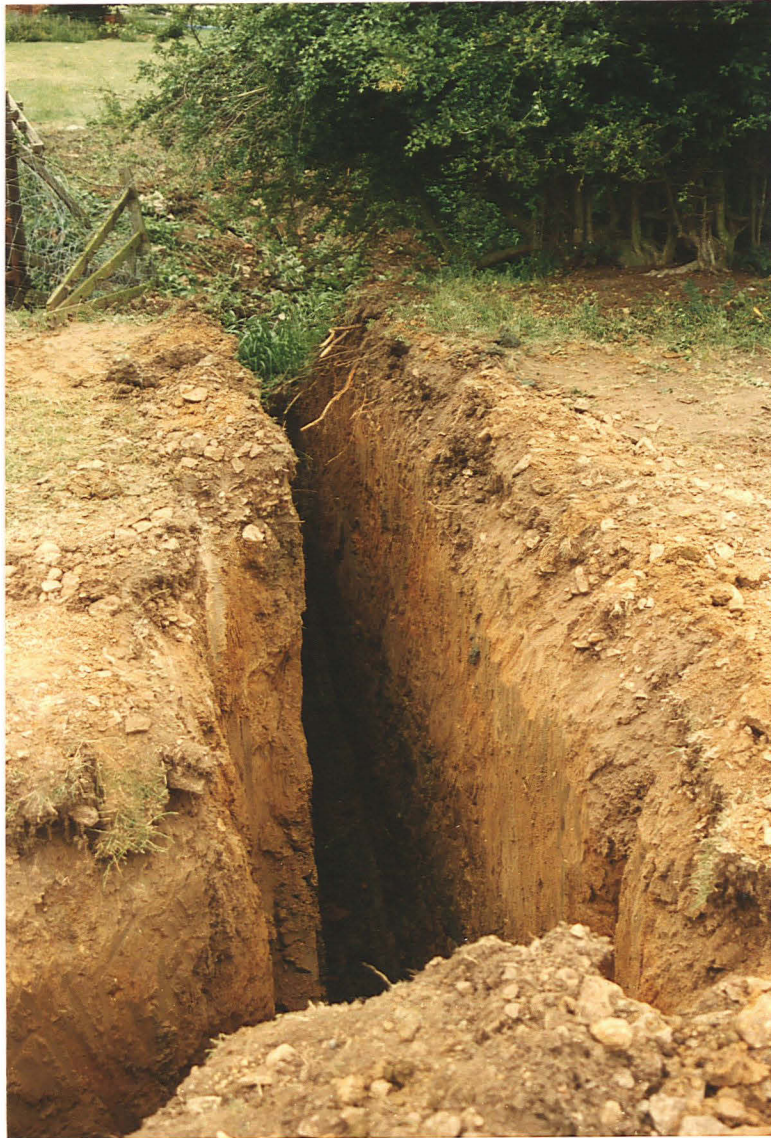
Pl. 11. View of the deeper pipe trench south of the stream crossing during excavation. The thick orange sandy clay with gravel layer overlies darker deposits (looking north).
