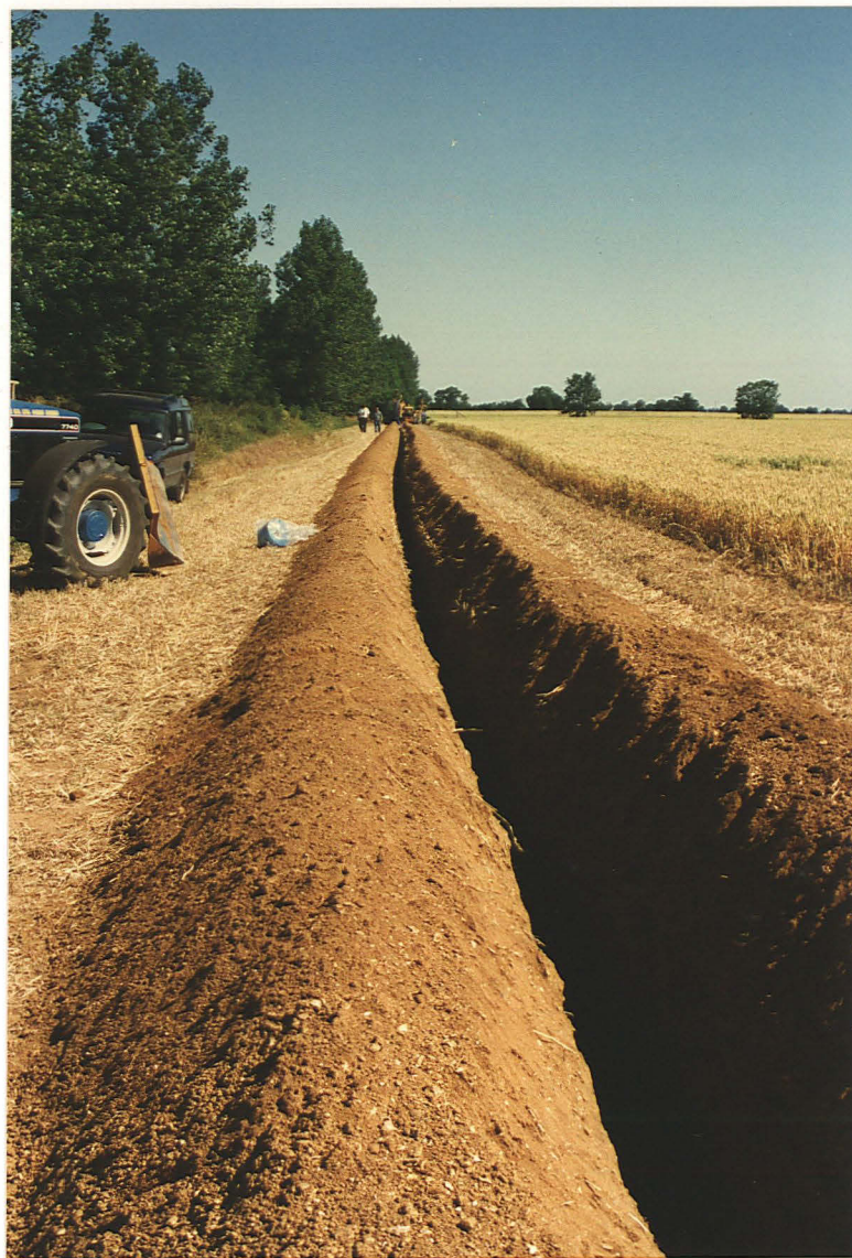
PI. 30. Position of the pipe trench in Morton parish, adjacent to the hedge of a removed railway line (looking north).
