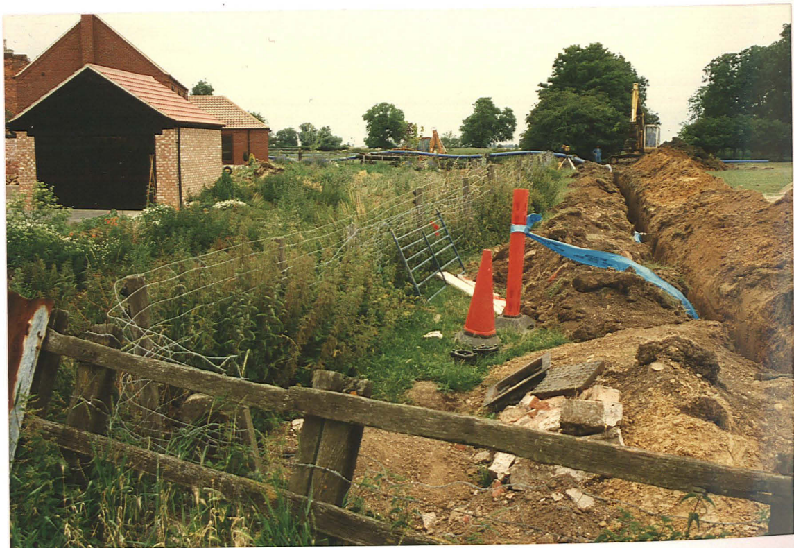
Pl. 2. The monitored pipe trench at Dyke, showing the position of the Car Dyke stream and the redeveloped farmyard site south of the stream. Ditch 1 crossed the trench behind the red cones. (Looking north).
