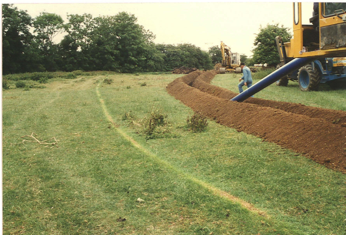
Pl. 22. Trenching north of the Car Dyke, using a land drainage machine to produce a narrower trench (looking south).
