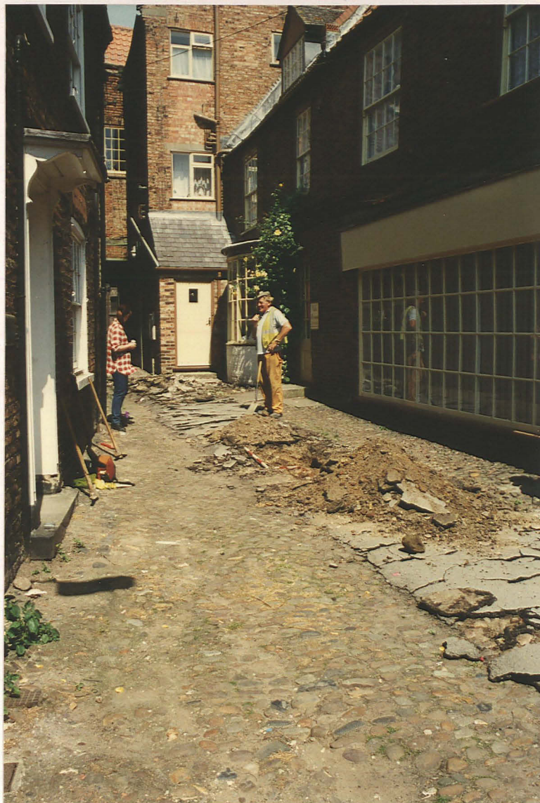
Pl. 1 Lindsey Court, view north, showing tarmac ready for removal. Trial excavation marked by small red and white photographic scale.
