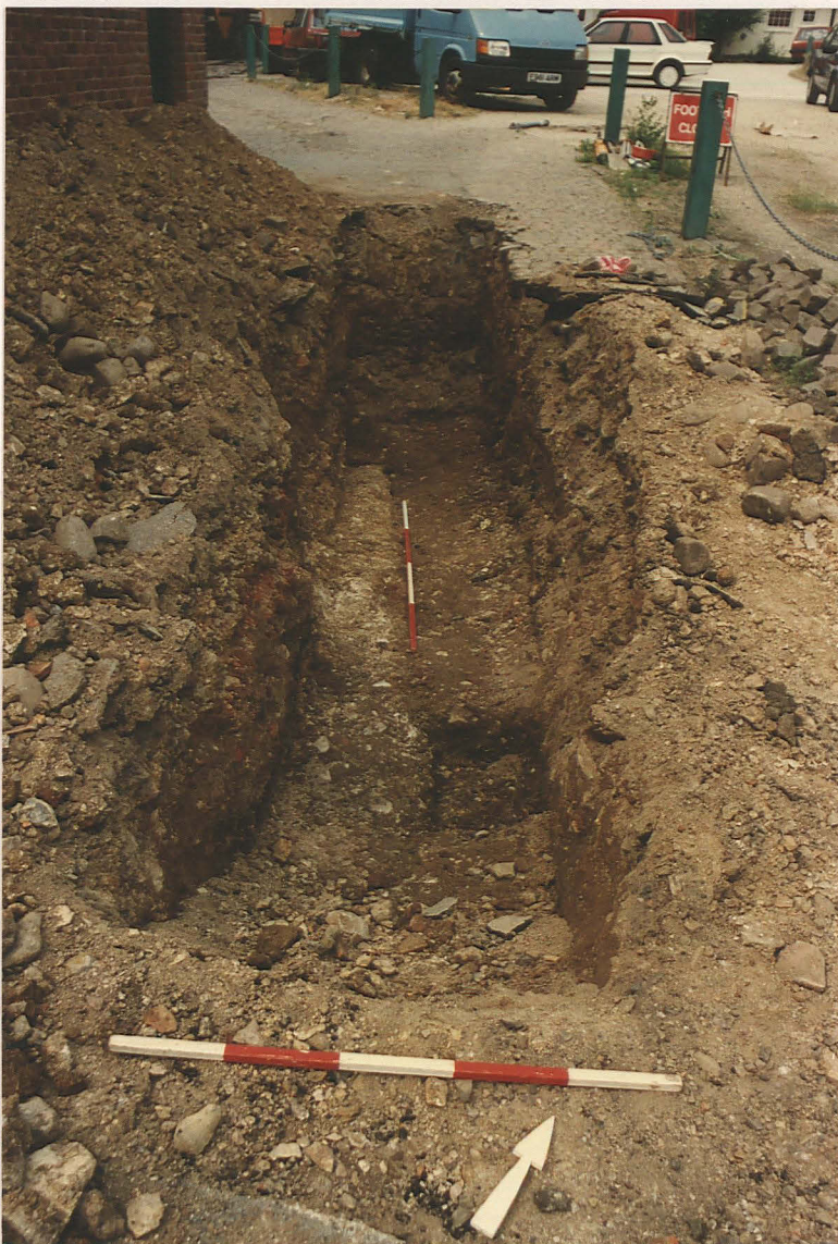
Pl. 5. Enlarged trench east of library excavated by JCB, view north, showing remains of Roman chalk foundation raft, left, and modern service trench, right.
